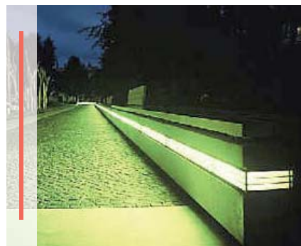
Recessed wall lights
