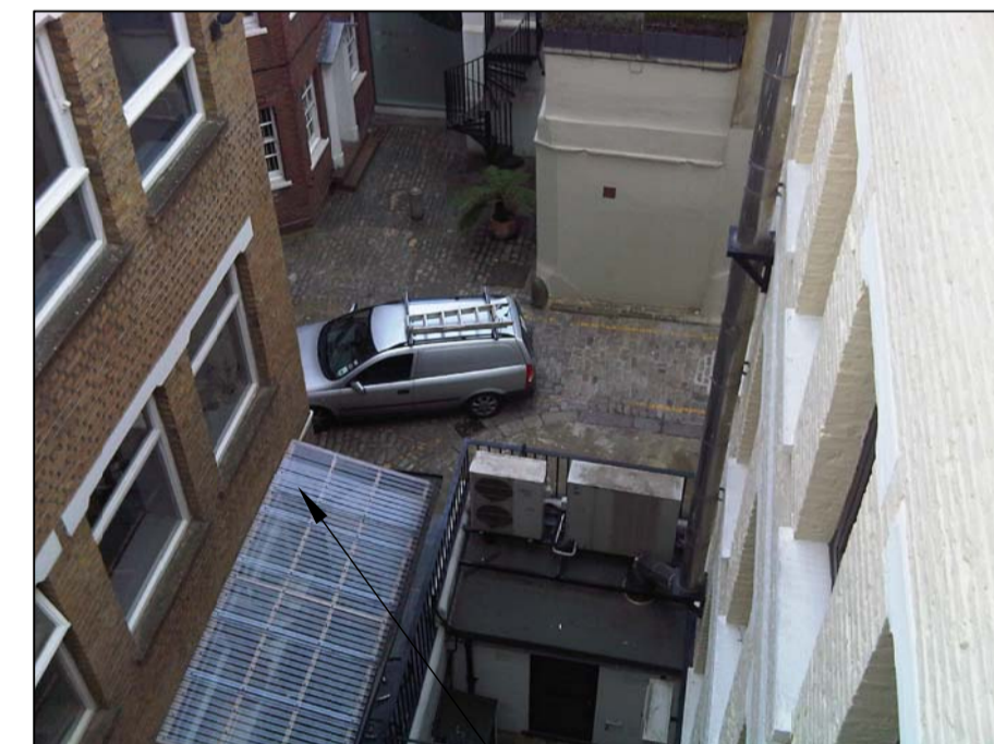
PHOTOGRAPH 1 LOCATION OF NEW GROUND FLOOR AIR CONDITIONING UNIT INSTALLED JULY 2013, REQUIRING RETROSPECTIVE PLANNING APPROVAL (AC UNIT IS WALL MOUNTED UNDER THE CANOPY - REFER TO ELEVATION A).
