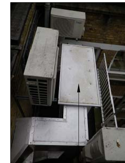
PHOTOGRAPH 2 LOCATION OF NEW SECOND FLOOR AIR HANDLING UNIT INSTALLED JULY 2013, REQUIRING RETROSPECTIVE PLANNING APPROVAL.
