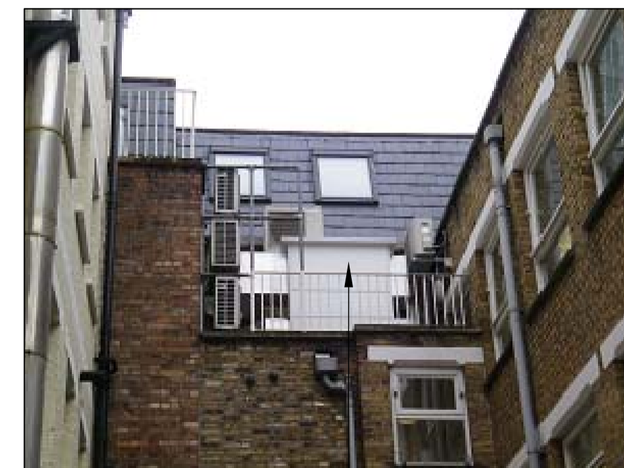
PHOTOGRAPH 3 LOCATION OF NEW SECOND FLOOR AIR HANDLING UNIT INSTALLED JULY 2013, REQUIRING RETROSPECTIVE PLANNING APPROVAL.
