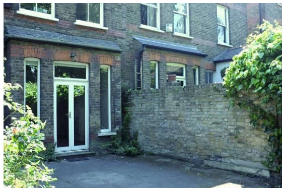
View showing the existing bay to be removed and garden wall to be heightened
