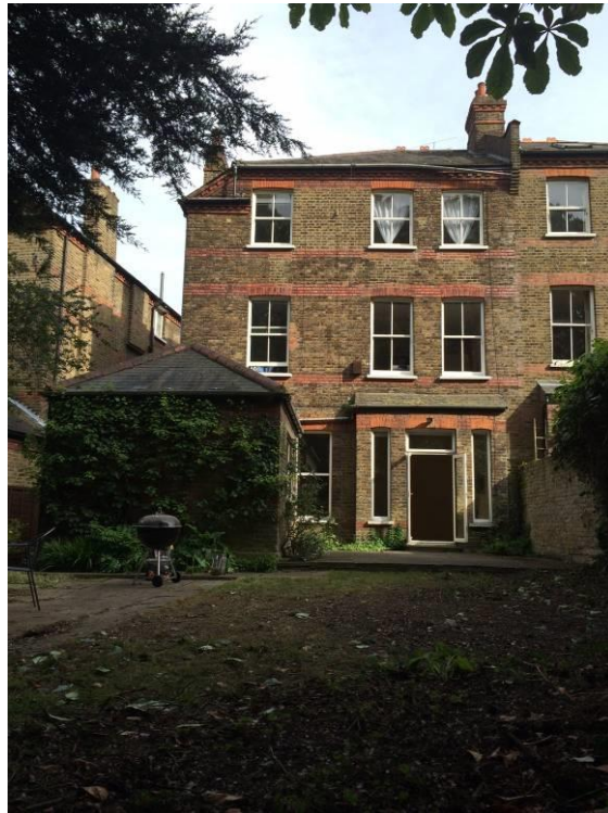
View from the garden, showing the existing rear extension and bay to be removed
