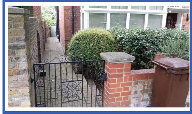
Plate 2: Side view along north west boundary of the property and showing storm water down pipes
