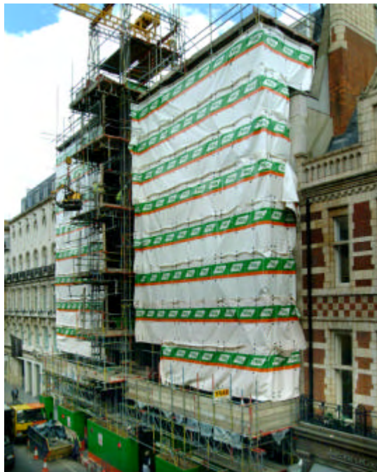
Figure 7: Building wrapped in monoflex sheeting to prevent escape of dust during construction
