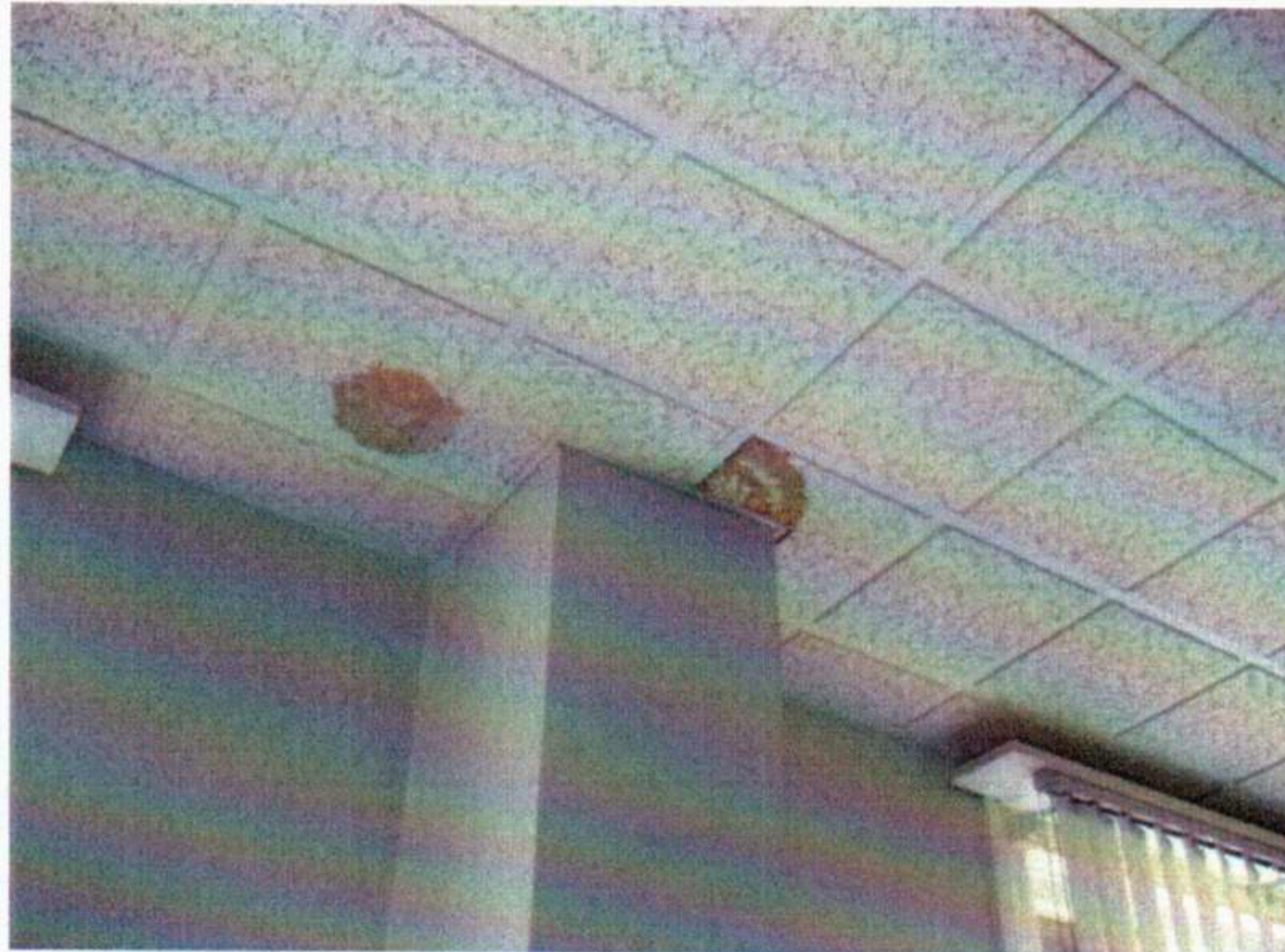
8. Evidence of dampness from parapet gutter outlet (?).
