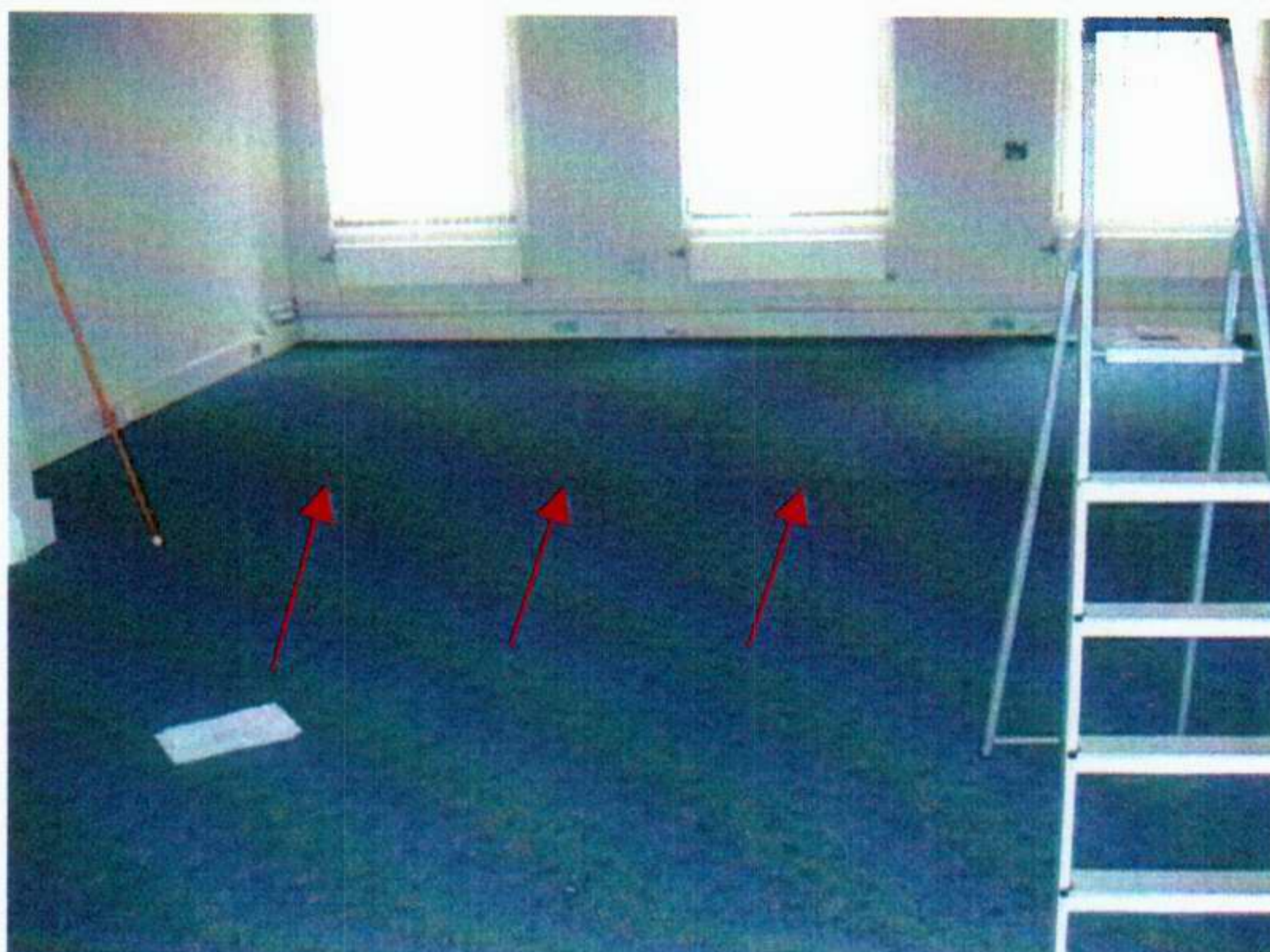
9. Slight hump in the floor at main supporting beam position.
