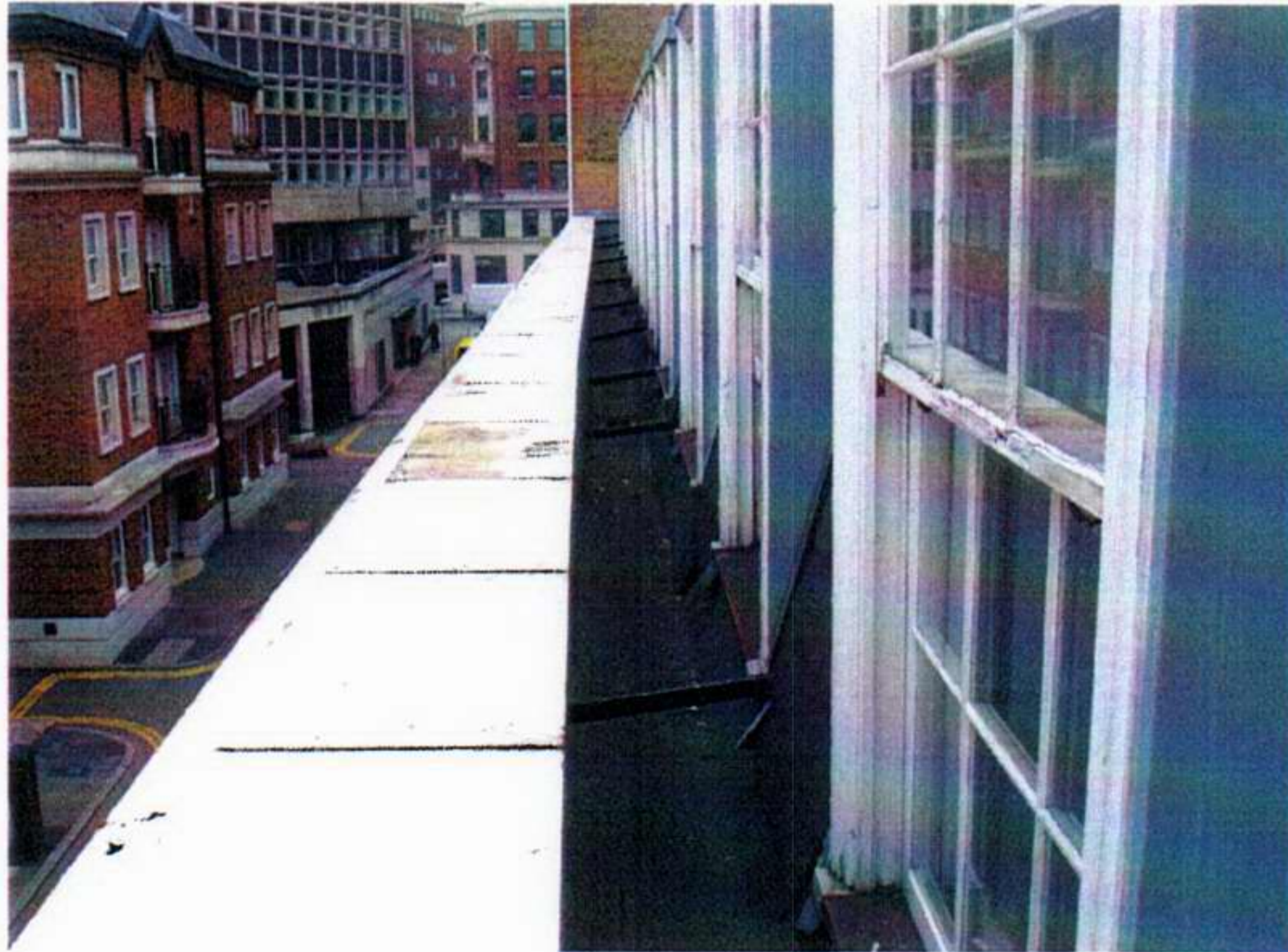
6. Slight distortion of front wall and dormer windows.
