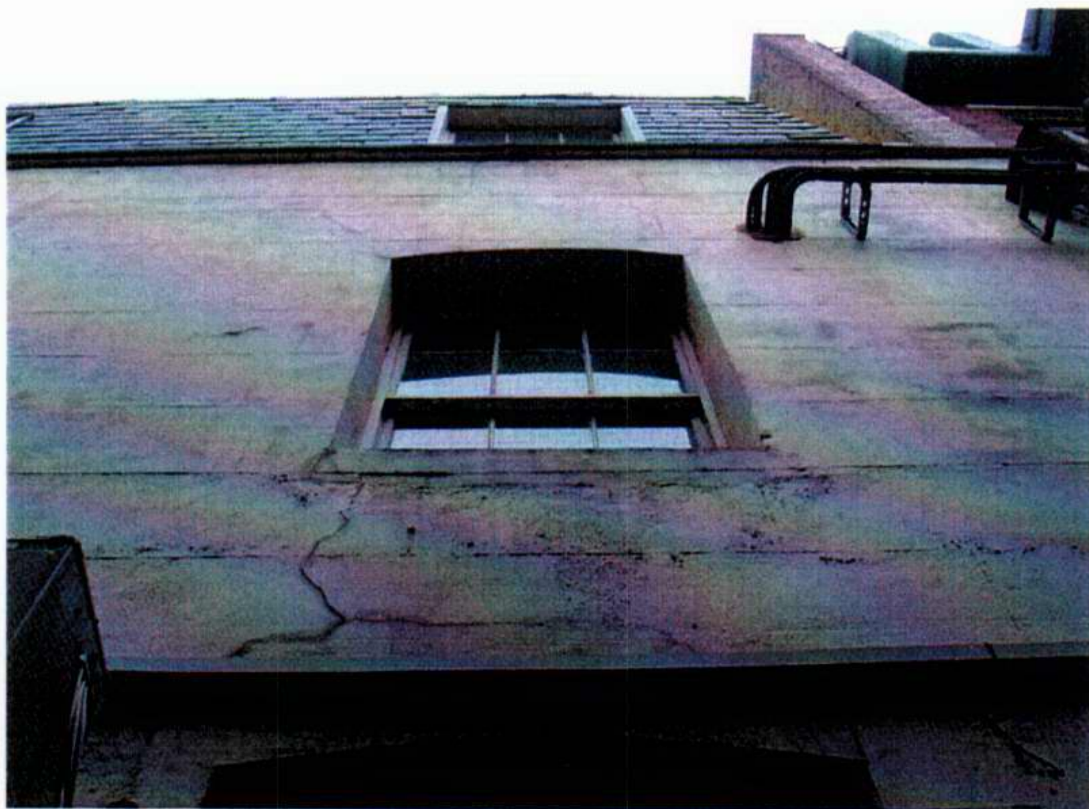
5. Hairline cracking of ashlar-render on rear wall.
