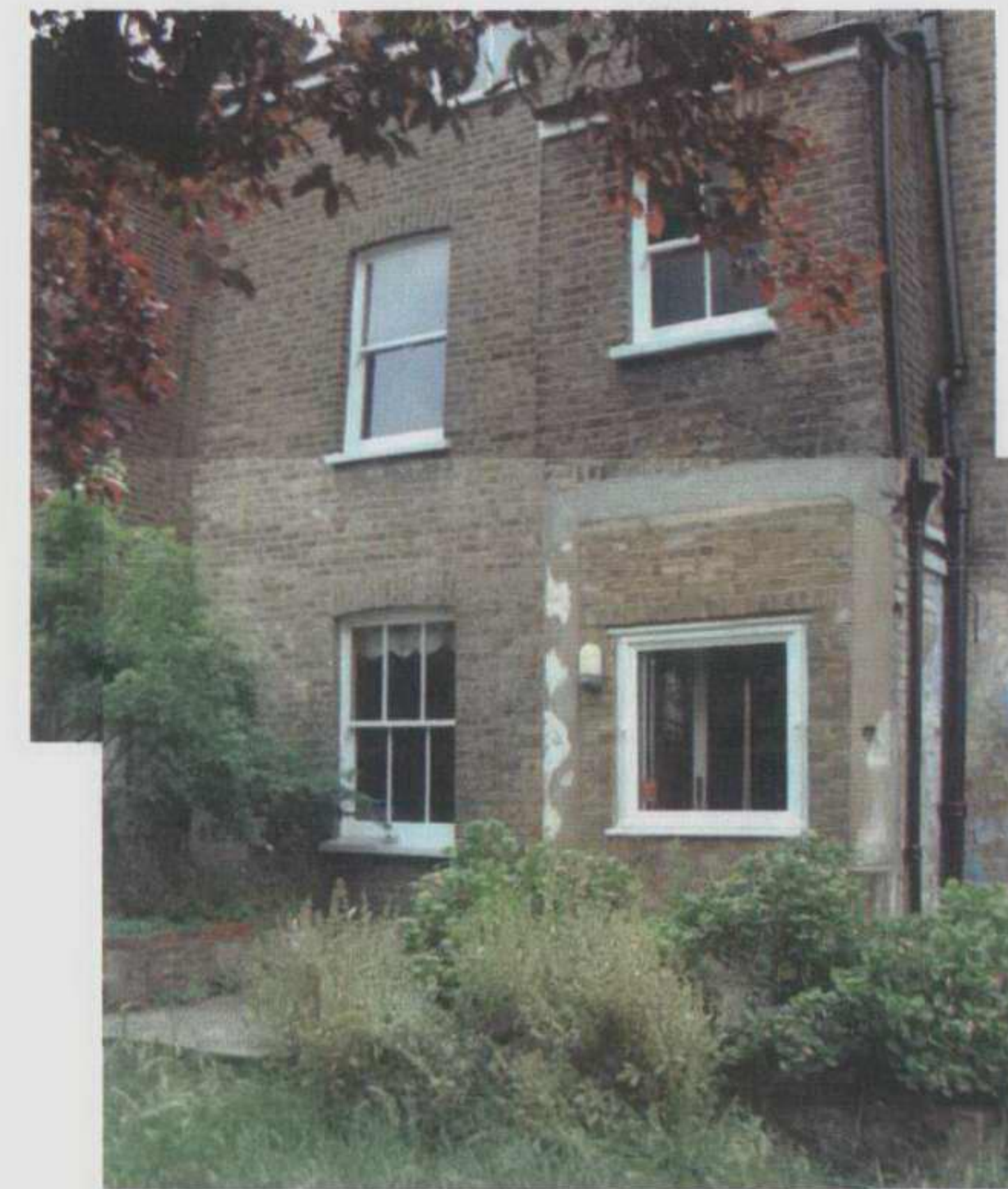
View of rear elevation showing existing extension repaired in the 1970s? and now structurally unsound
