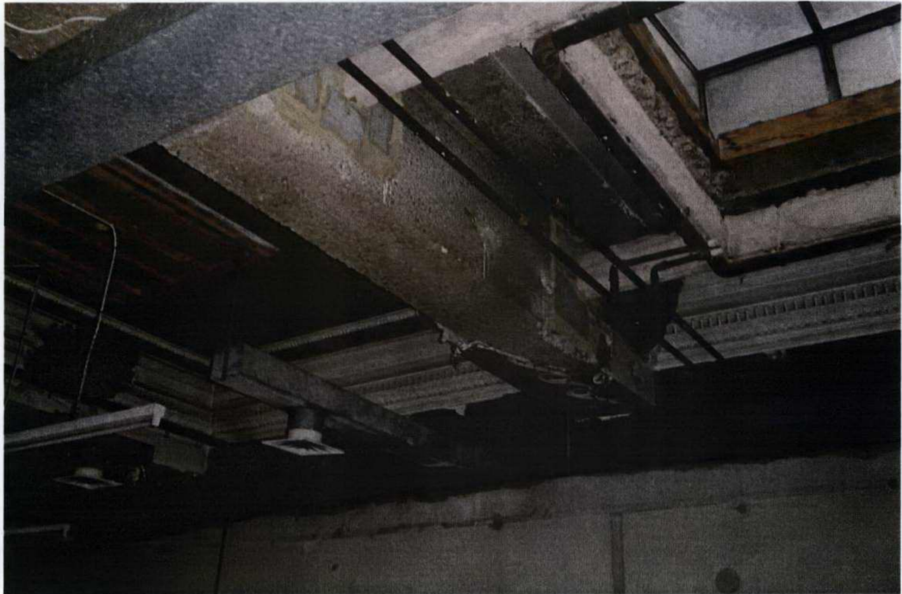
Ref: 004 – View on Damaged Ornate Down Stand Beams
