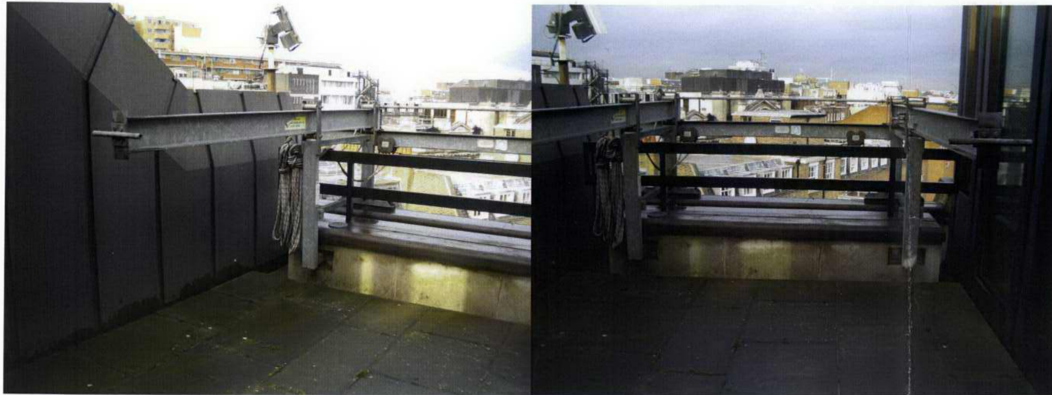
VIEWS OF WINDOW CLEANING APPARATUS ON REAR (NORTH) ROOF AREA - TO BE REMOVED
