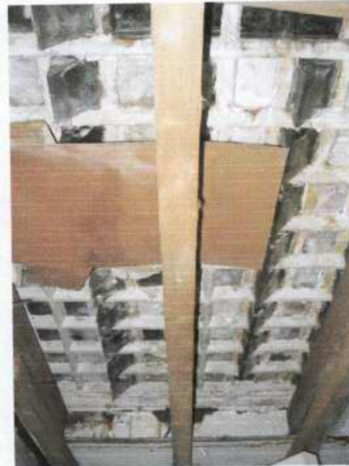
06. View of existing entrance bridge in hazardous conditions. Proposed to be re-build as existing.
