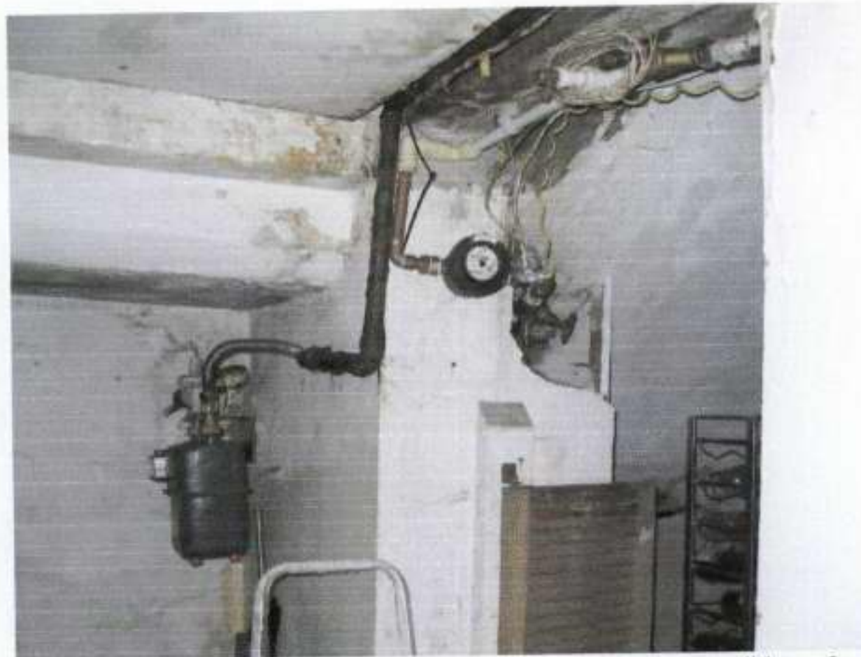
05. View of existing vaults showing poor / hazardous condition of services mains.
