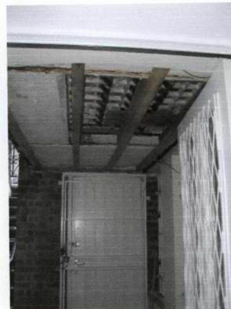
08. View of existing patio showing entrance bridge in poor conditions.
