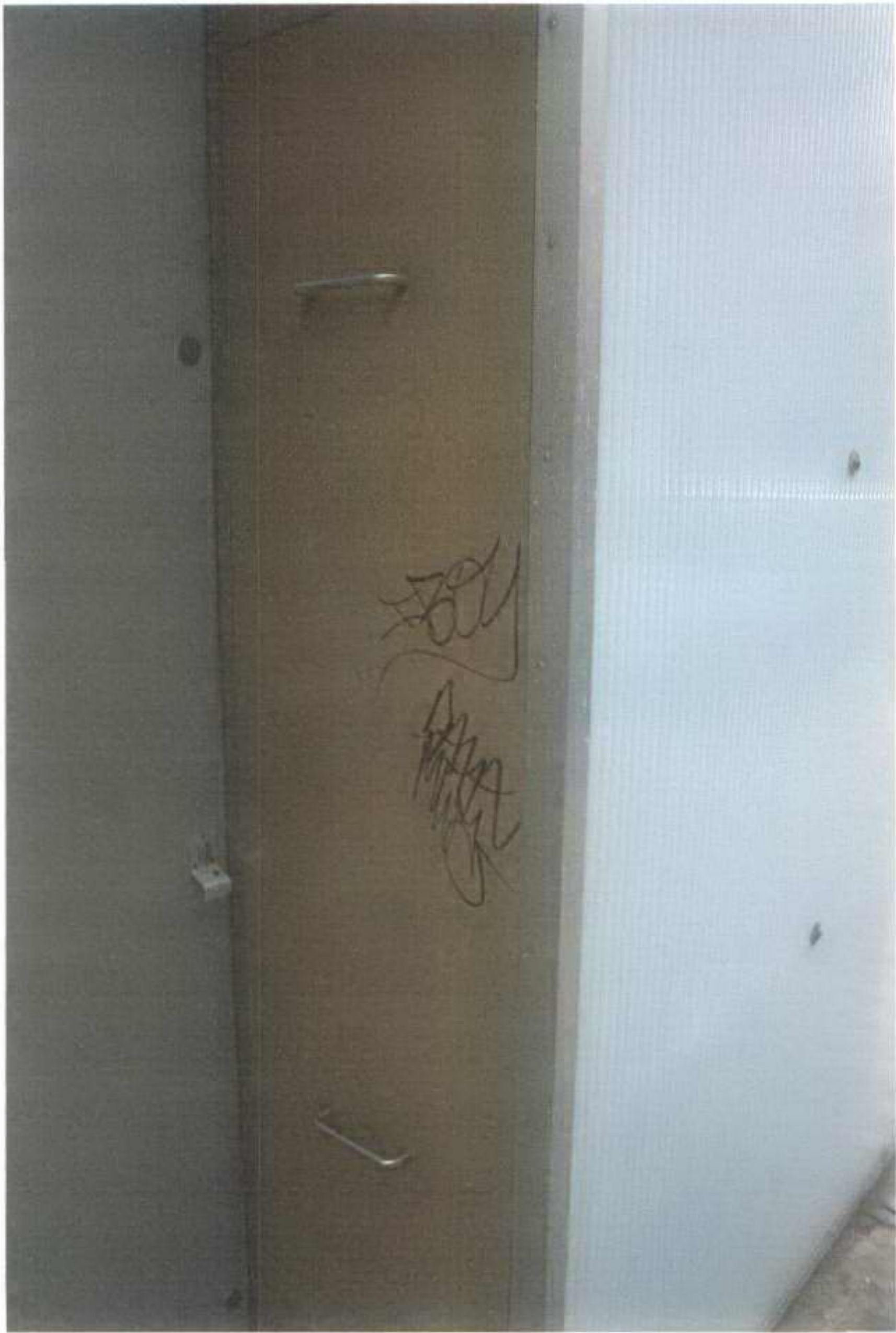
GRAFFITI BY THE ENTRANCE DOOR TO 1 BETTERTON STREET
