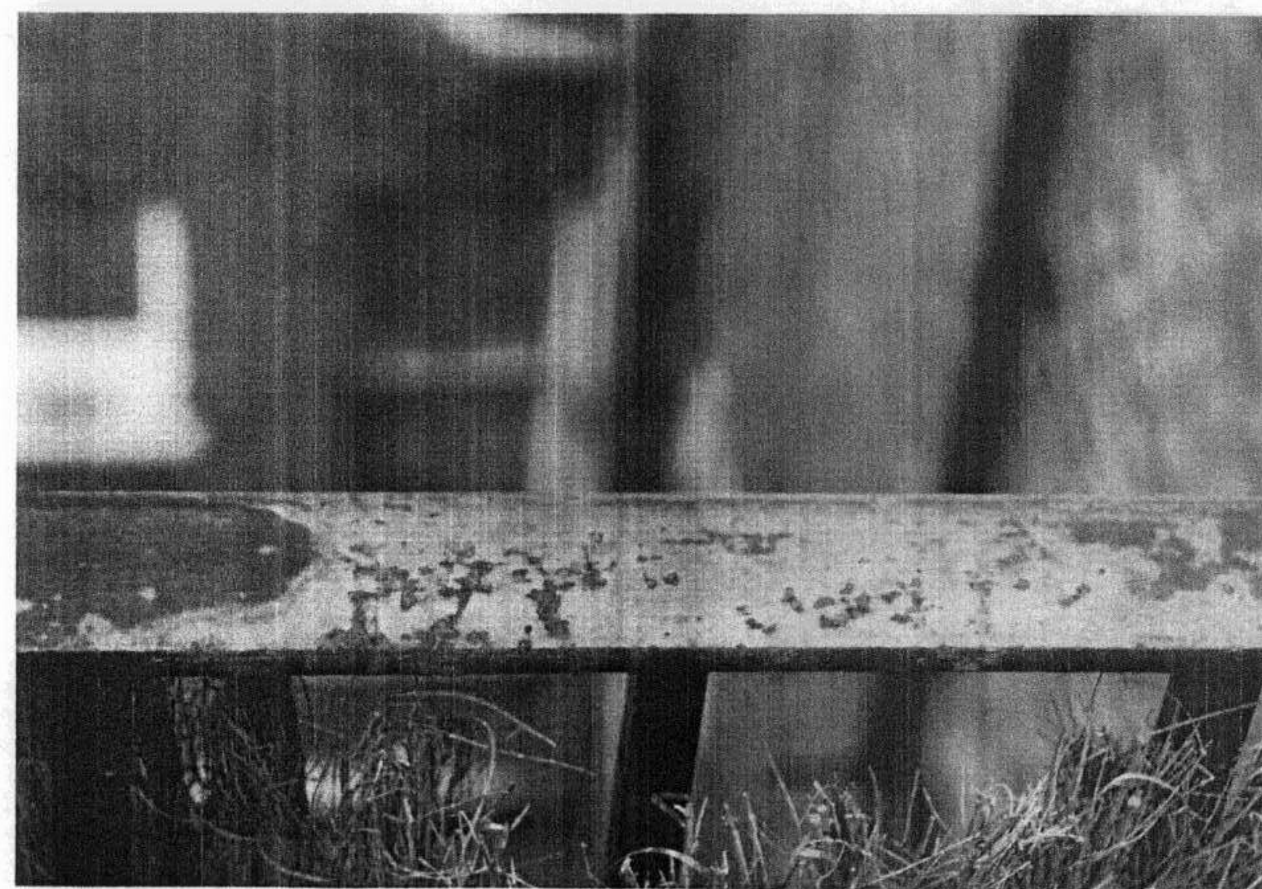
SIGN OF RUST ON RAILINGS INDICATE AGE ↗
