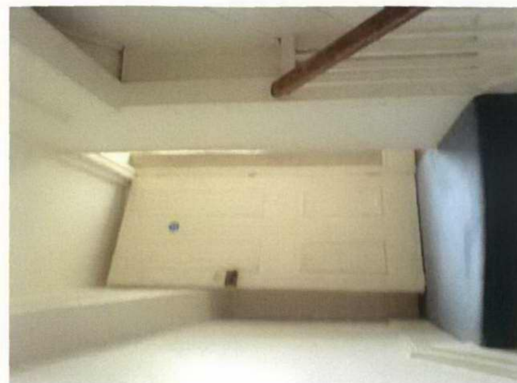
1. View to half landing door
