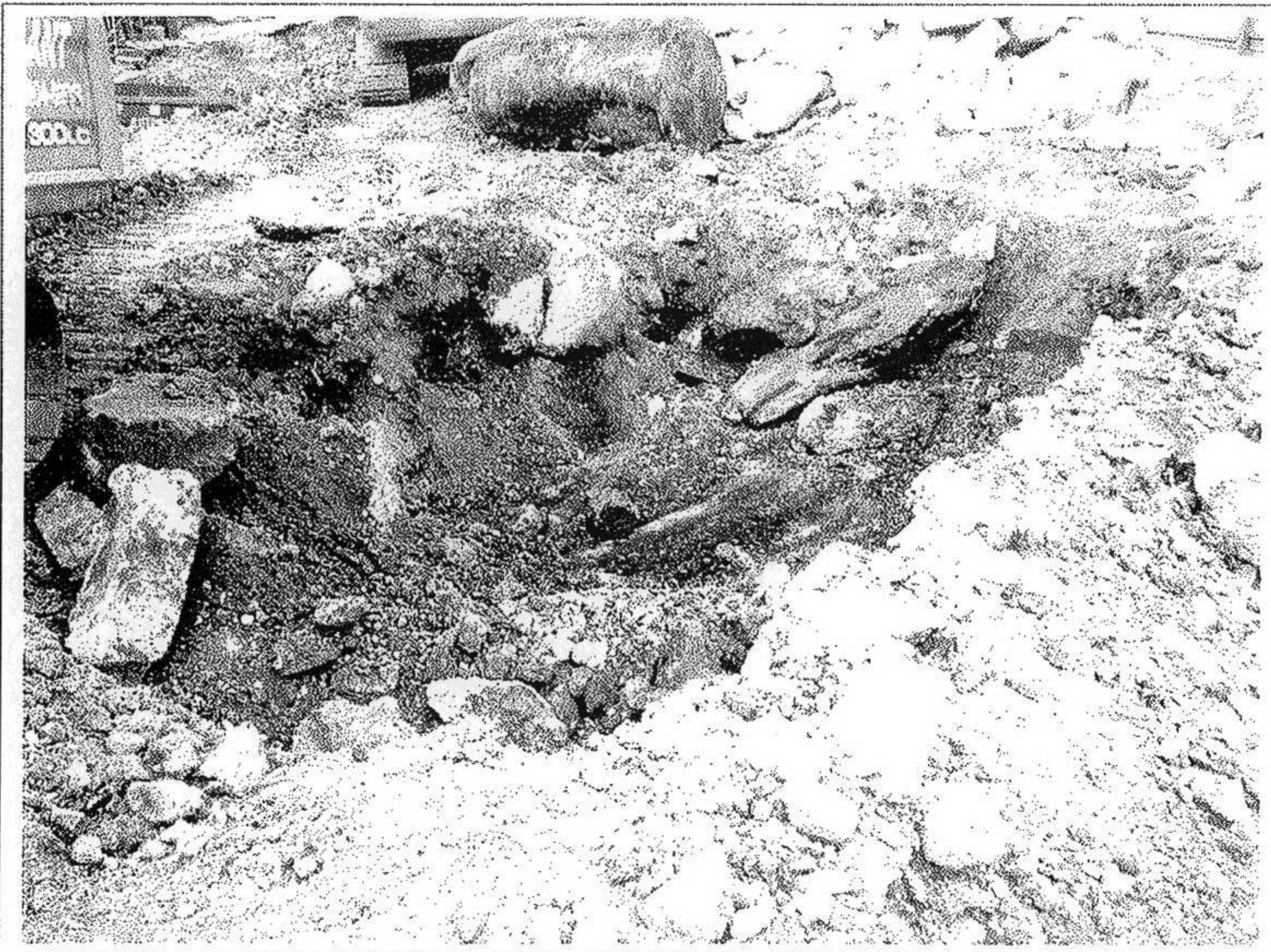
Photo 7: Staining on concrete base beneath tanks 7 and 8.
