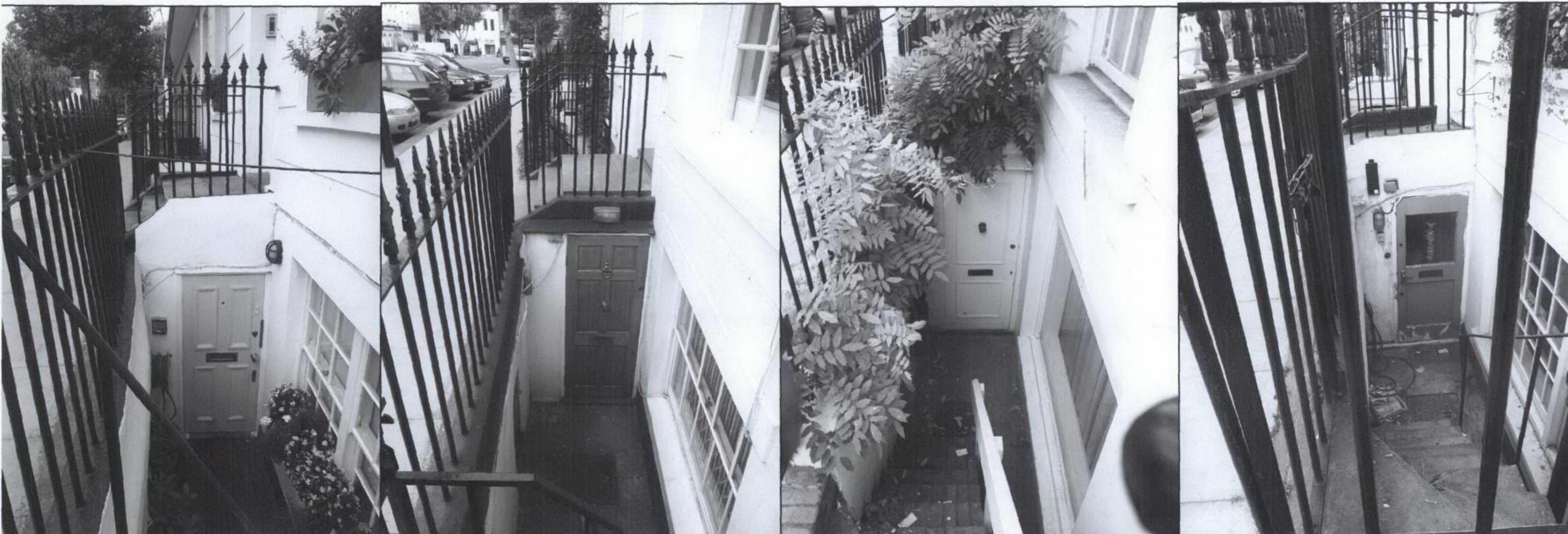
PROPERTIES ALONG ALBERT STREET WHICH HAVE RE-POSITIONED THE FRONT DOOR AT LOWER GROUND LEVEL
