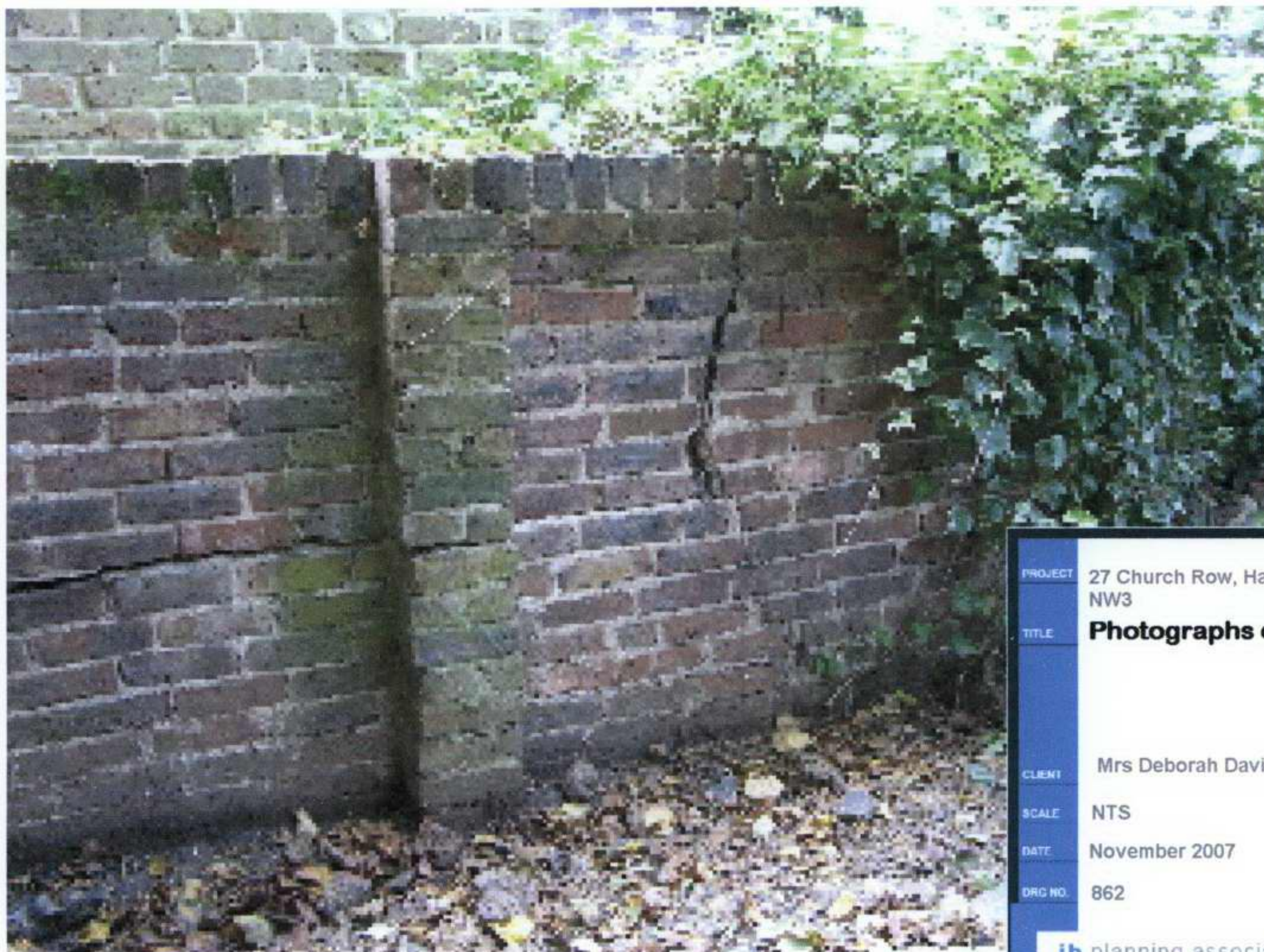
Photo 4: Rear boundary wall – detail of structural failure.
