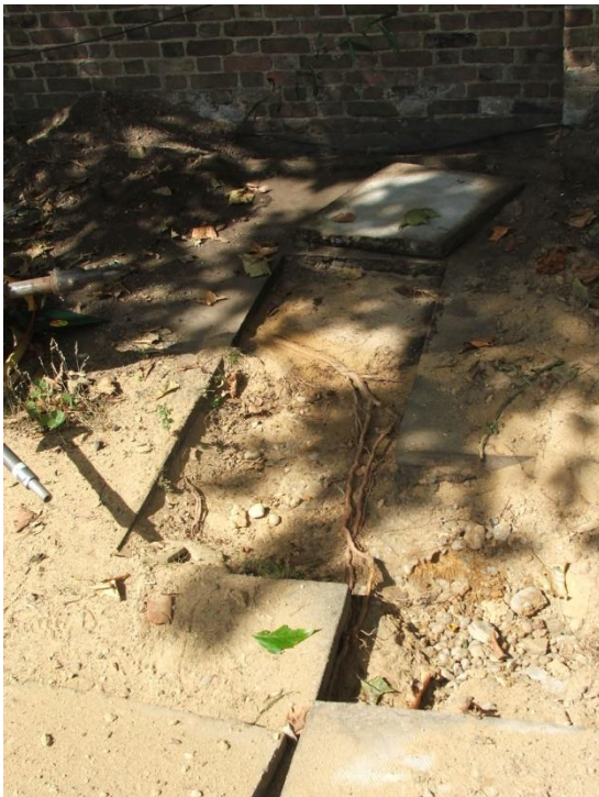
Plate 6: (photo 3365) showing lifted paving in relation to T16
