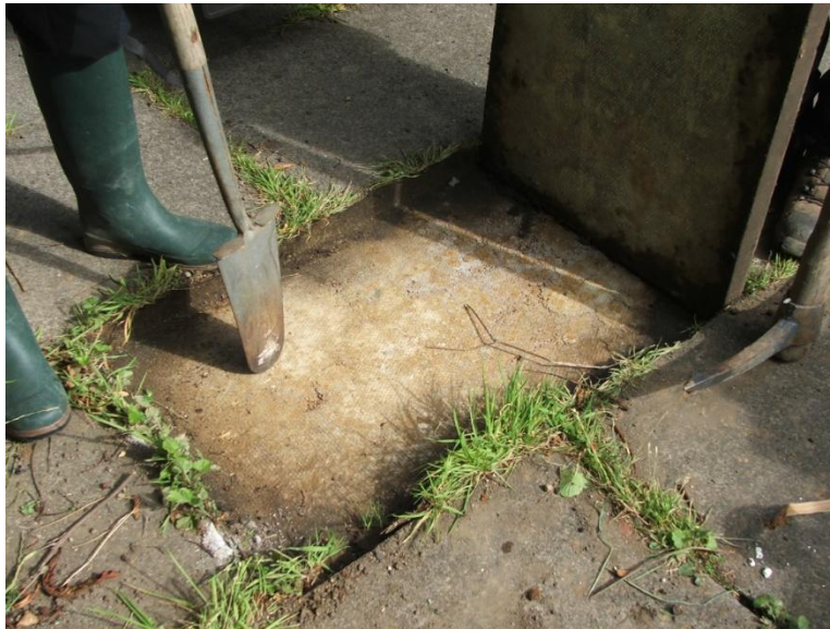
Plate 1: (photo 3393) showing lifted paving relating to tree T5
