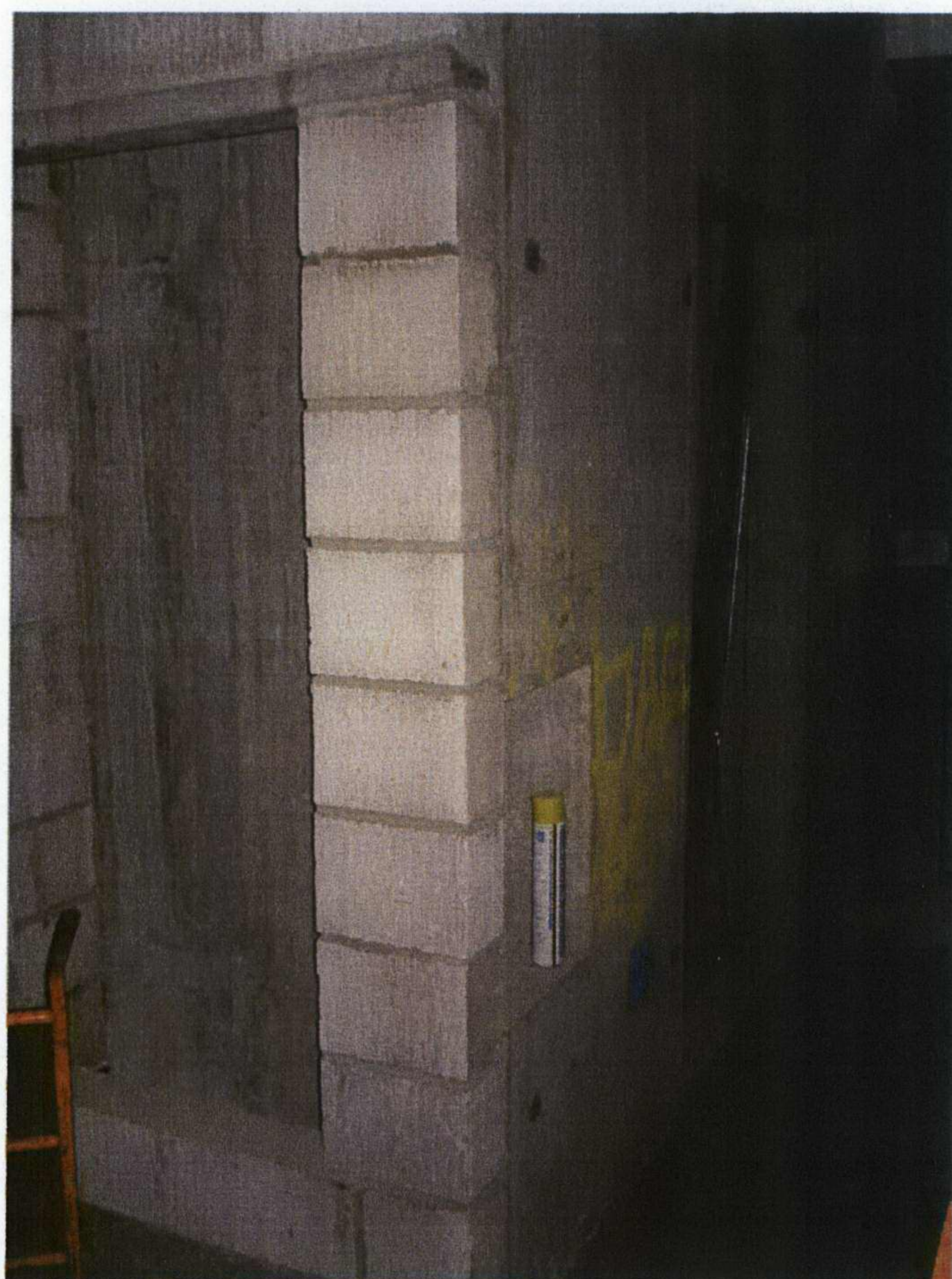
2. Lobby Area - Dry Riser Outlet position on Lift Core, low level (South).
