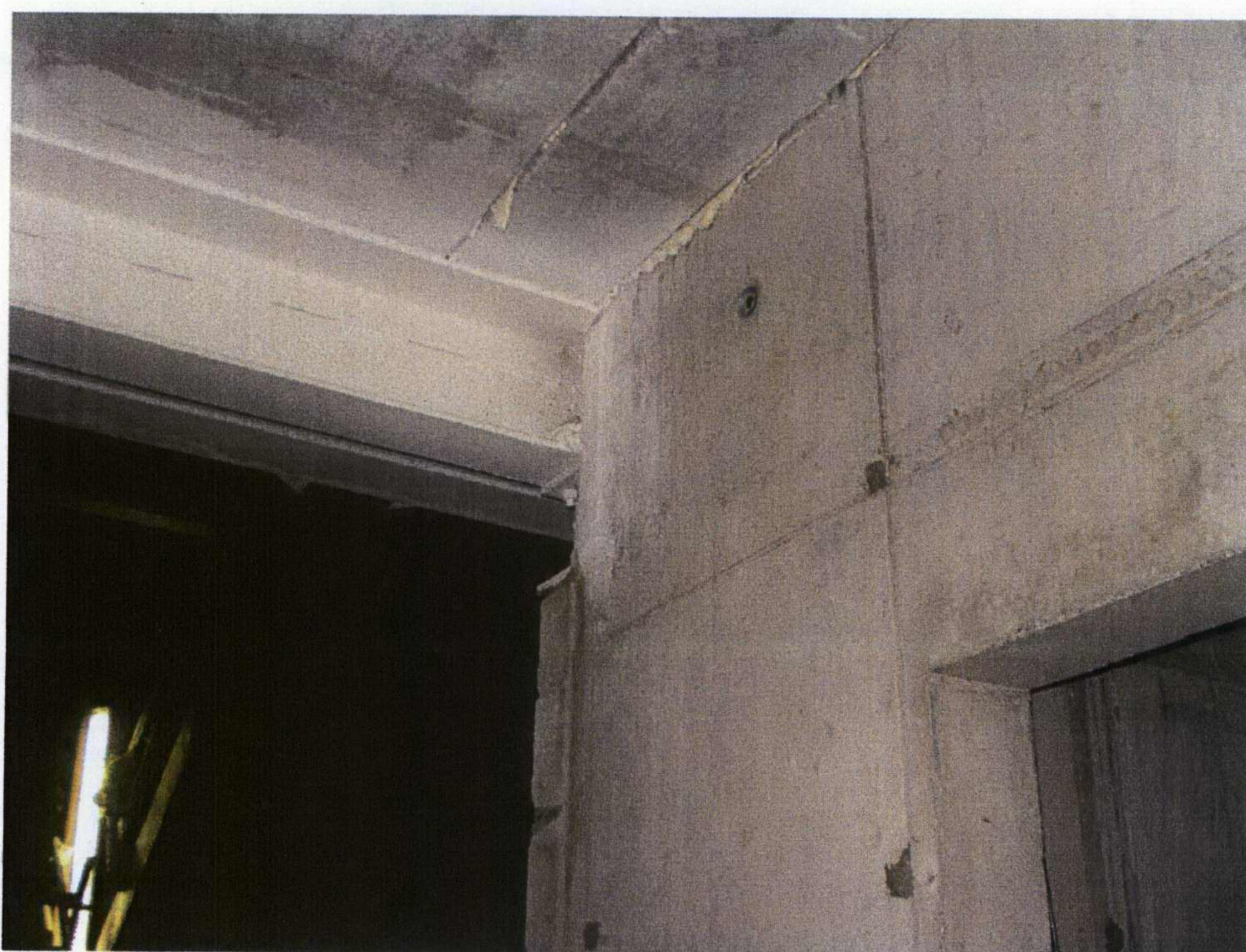
4. Lobby Area - Dry Riser Outlet position on Lift Core, high level (North).
