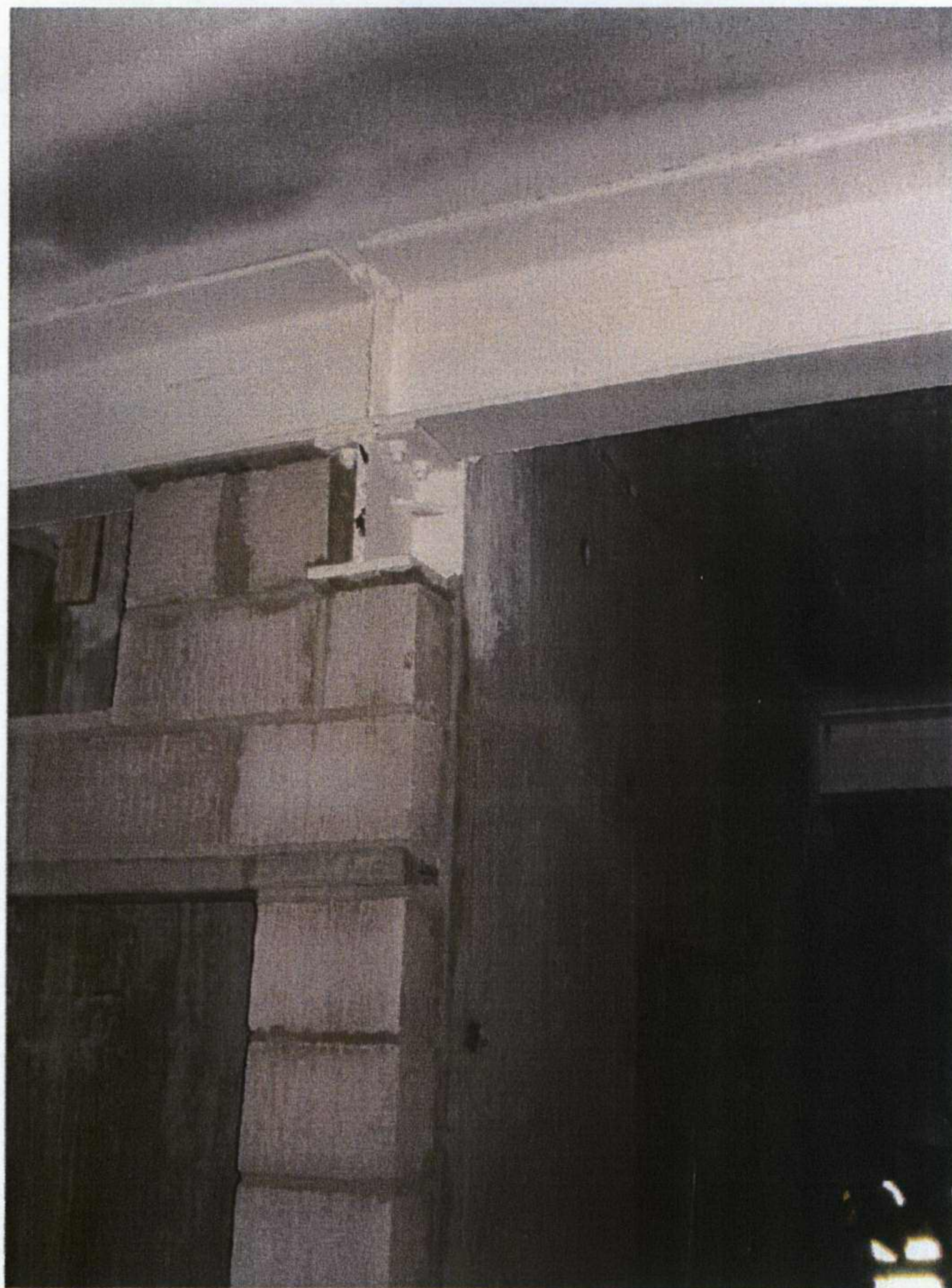
1. Lobby Area - Dry Riser Outlet position on Lift Core, high level (South).
