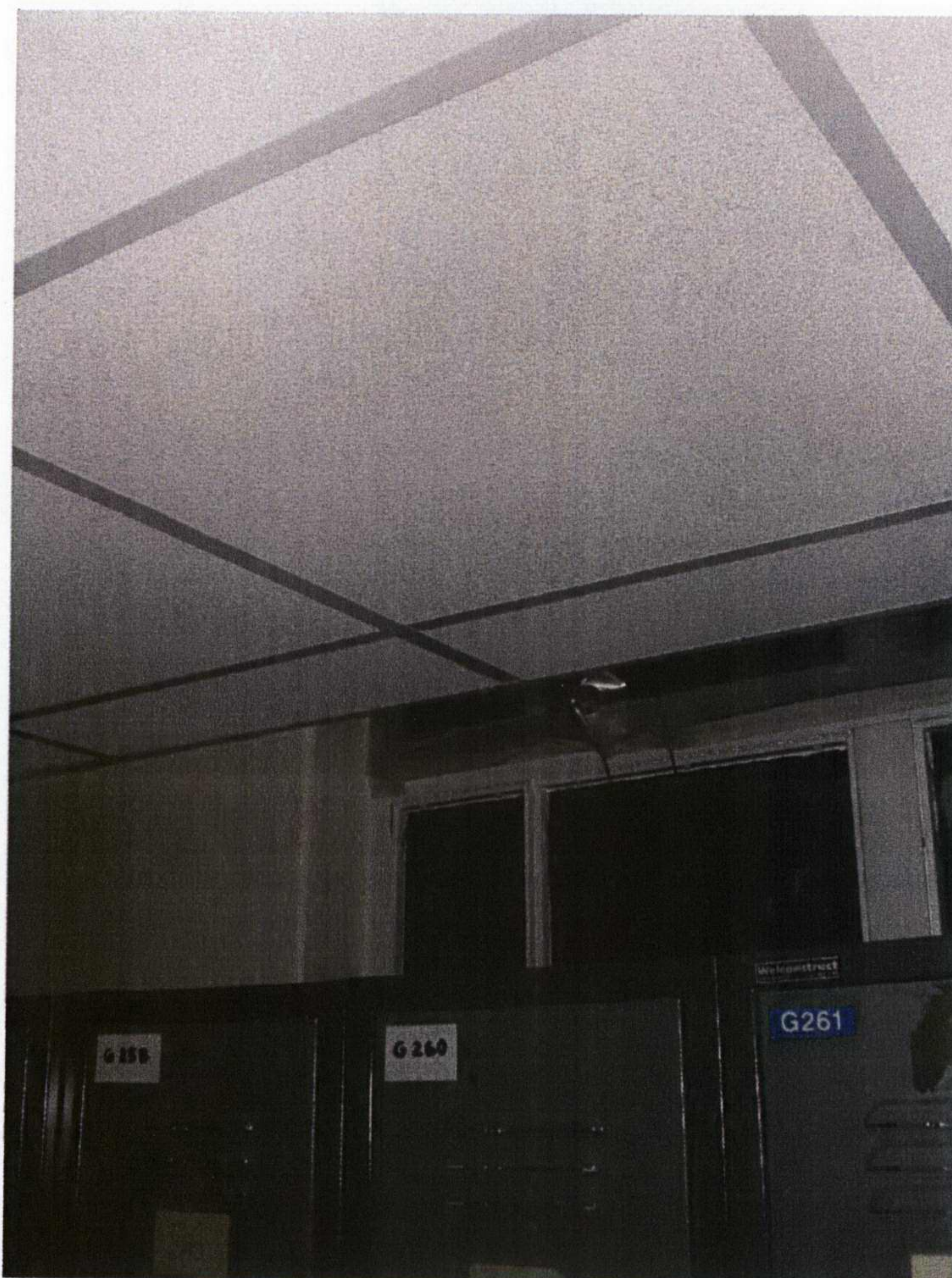
7. Hall between Lobby Area & computer room - Dry Riser penetration, Internal window W/LG/W/04 (East).
