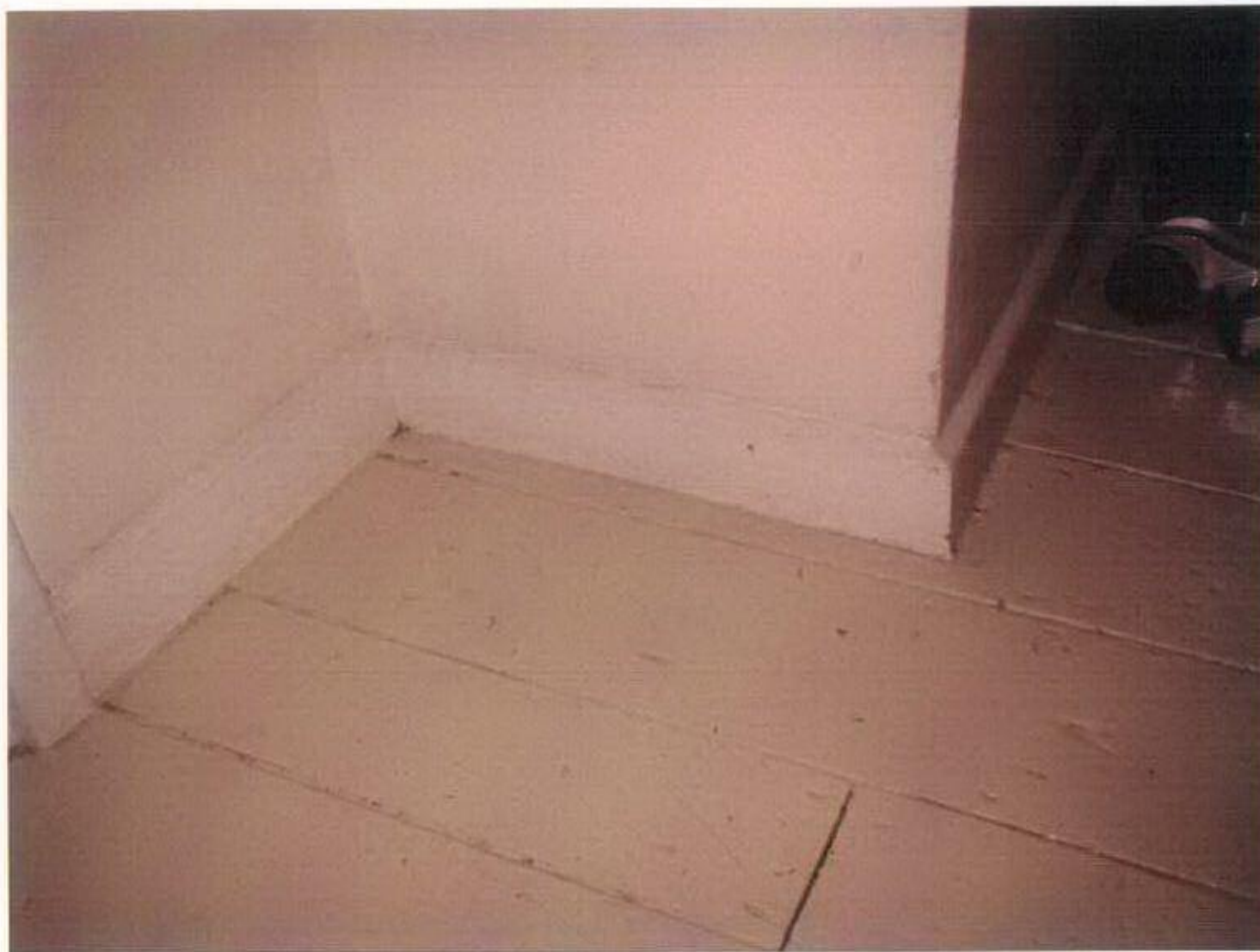
Photograph No. 14 – Skirting board to south wall and chimney breast Living Room - 29 Buckridge Building
