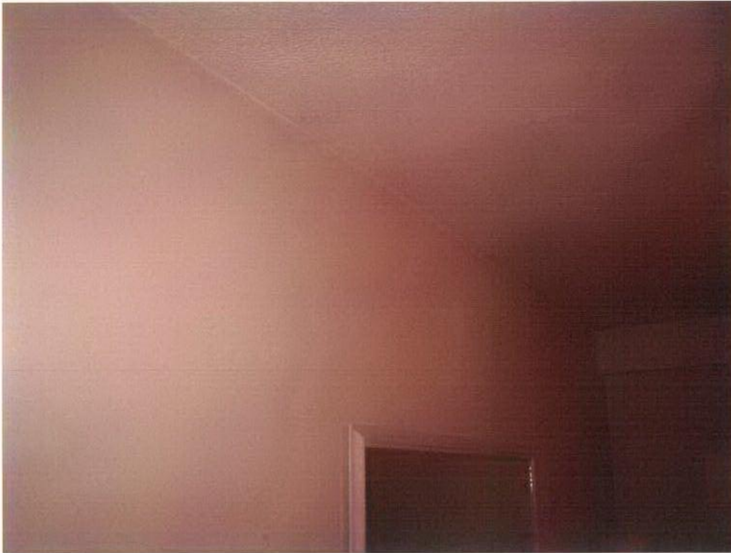
Photograph No. 12 – Junction of ceiling and north wall Living Room - 29 Buckridge Building
