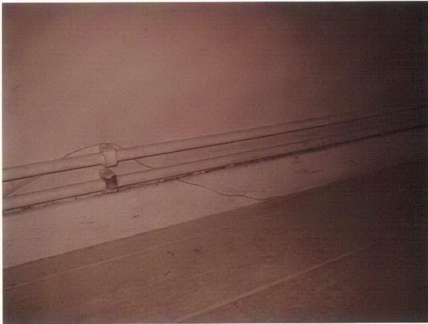
Photograph No. 13 – Skirting board to west wall Living Room - 29 Buckridge Building
