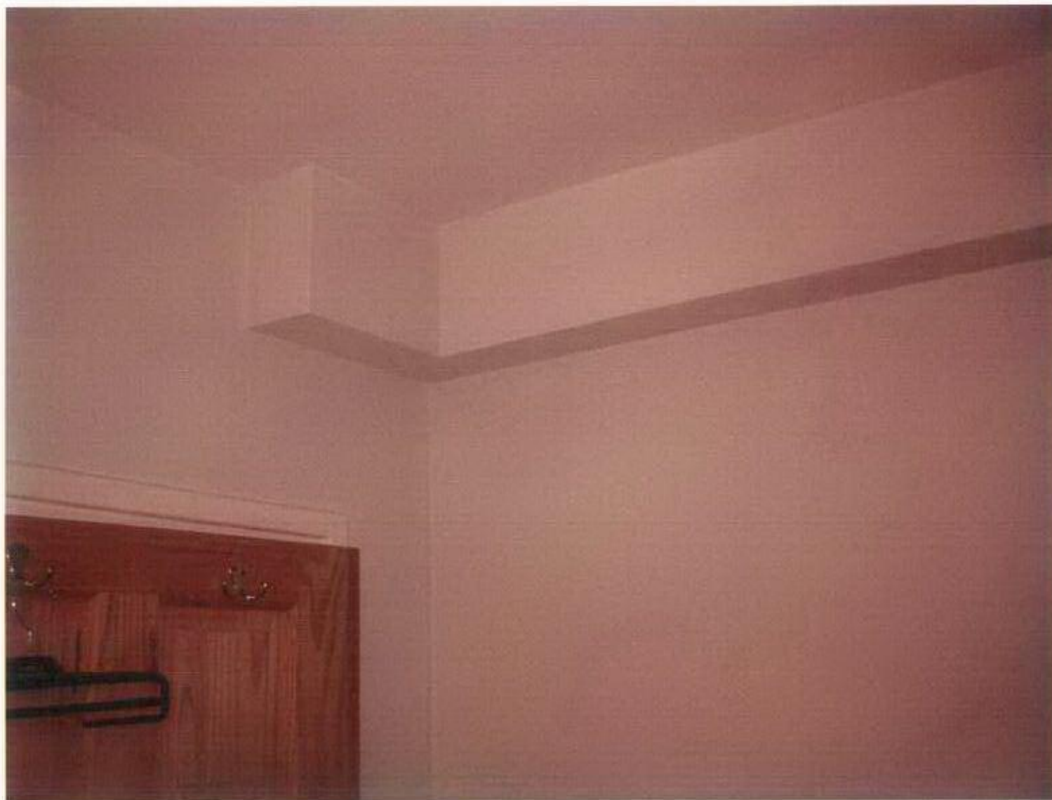
Photograph No. 16 – Junction of Ceiling, “boxing” around pipes and north & east walls Bedroom - 29 Buckridge Building
