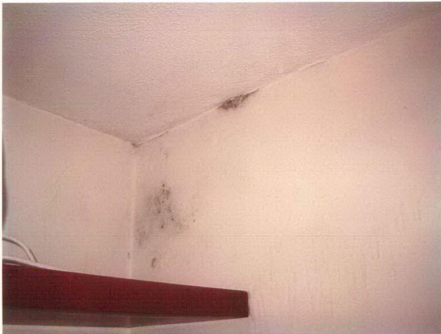
Photograph No – 11 Junction of ceiling and south & west walls Living Room - 29 Buckridge Building
