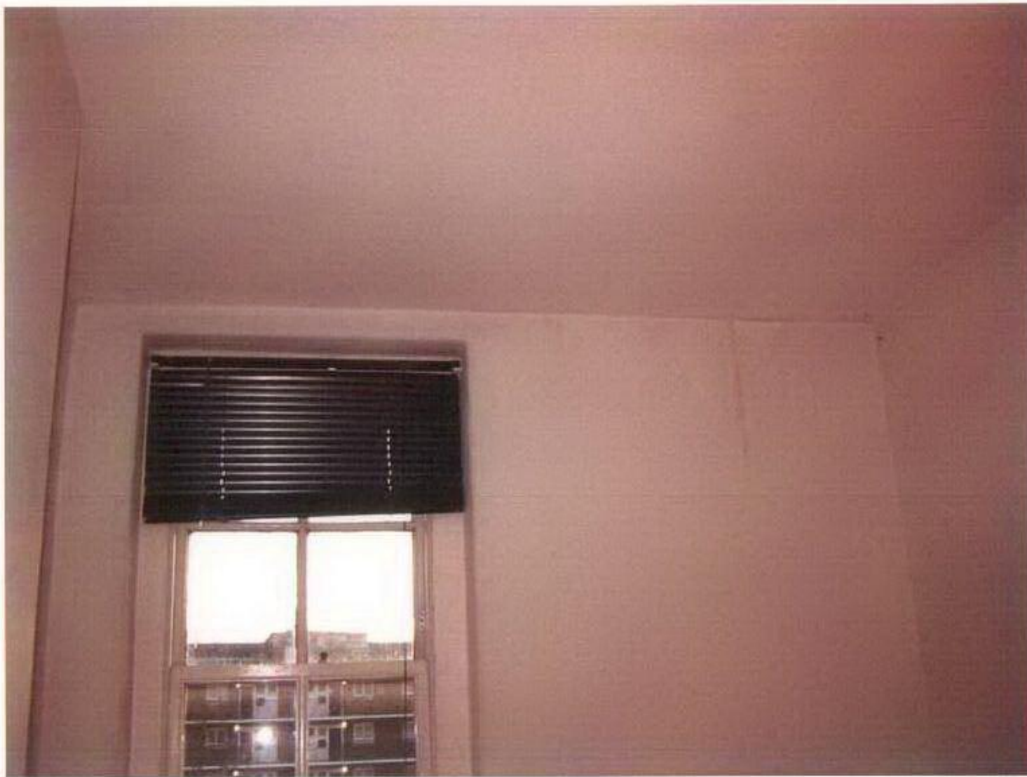
Photograph No. 15 – Junction of ceiling and west wall Bedroom - 29 Buckridge Building
