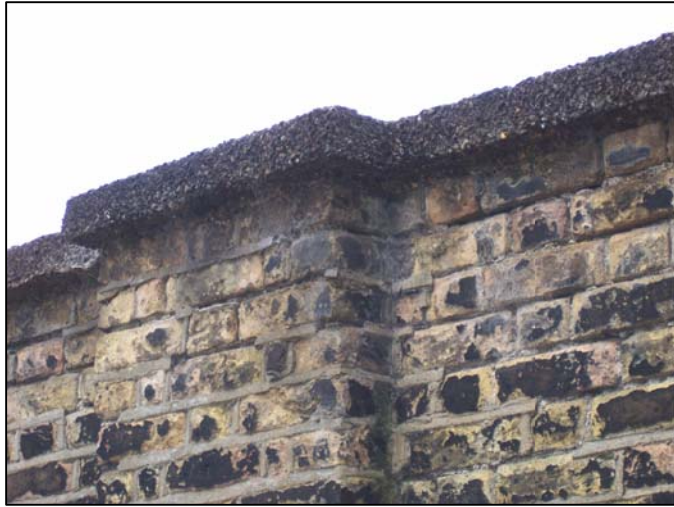
Photographs of the Modern Roughcast Coping Note: Poorly detailed, inadequate overhang, no drip throat, flat top with no weathering, no dpc.
