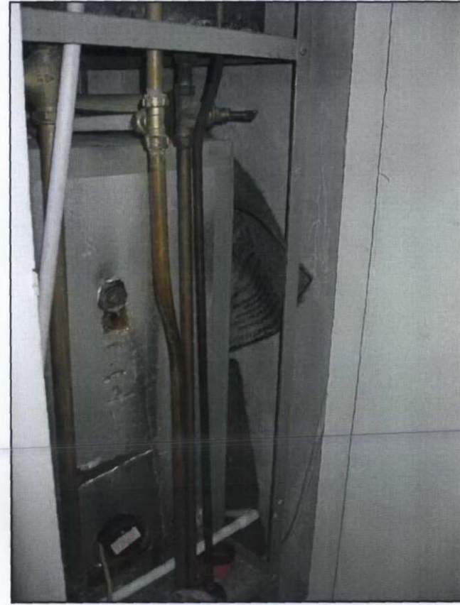
09 EXISTING HOT WATER HEATER
