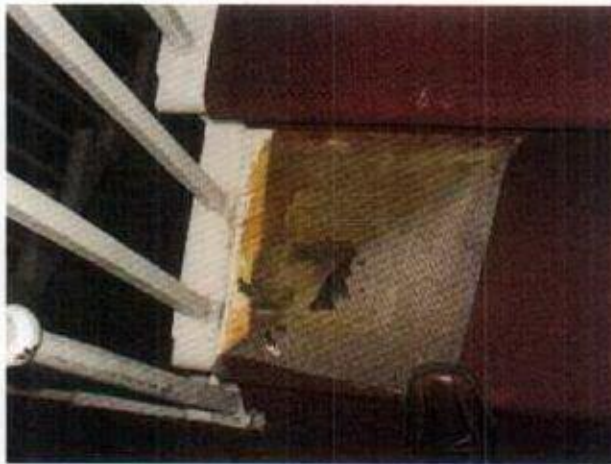
Photograph 2: Diagonal cracking to top of cantilever stone step.
