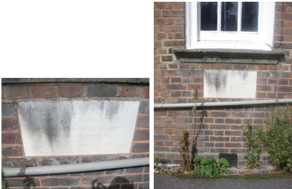
Image 2 – Stone Plaque No.2 to be removed and returned to the Contract Administrator. This item must not be damaged.
