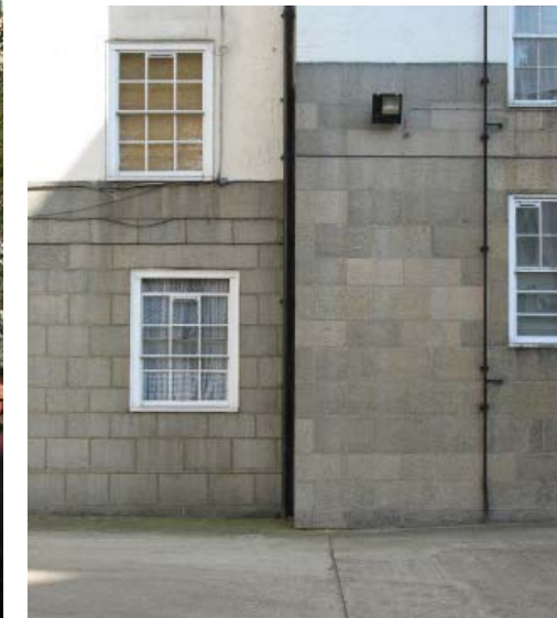
Subtle variations in colour in concrete blocks that form the plinth of Levita House
