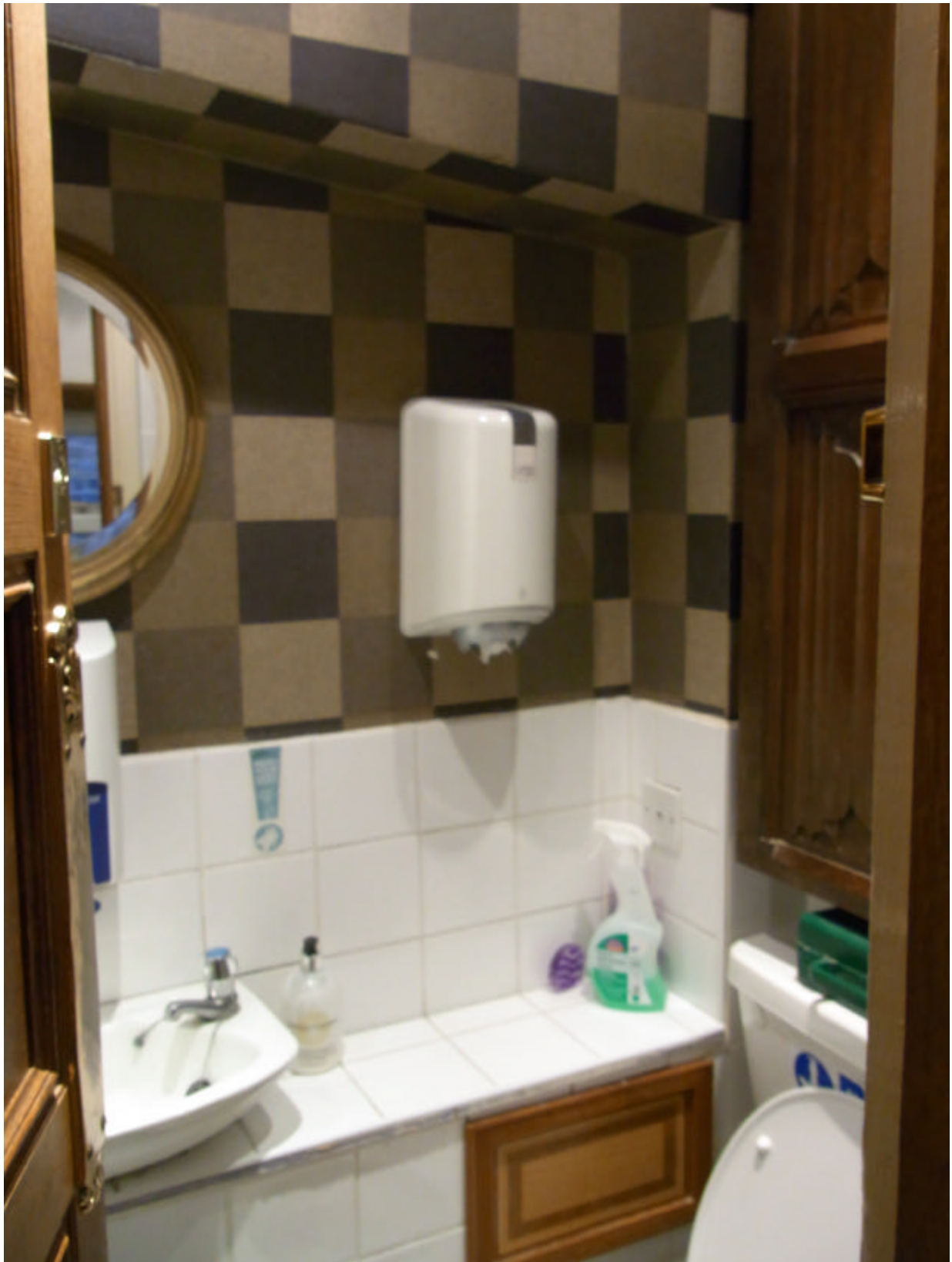
7. Existing WC. Partition on the right and bulkhead to be removed to form ensuite shower room.
