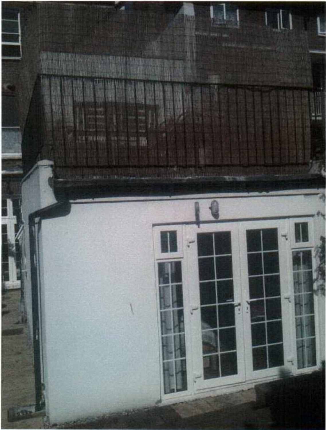
VIEW FROM THE GROUND FLOOR UP TOWARDS THE REAR OF THE TERACE SHOWING THE EXISTING HANDRAIL + BAMBOO SCREENS.
