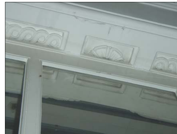
P10 PHOTOGRAPH PLASTER MOULDING TO UNDERSIDE OF ARCH OBSCURED BY HIGH LEVEL TIMBER FRAMING
