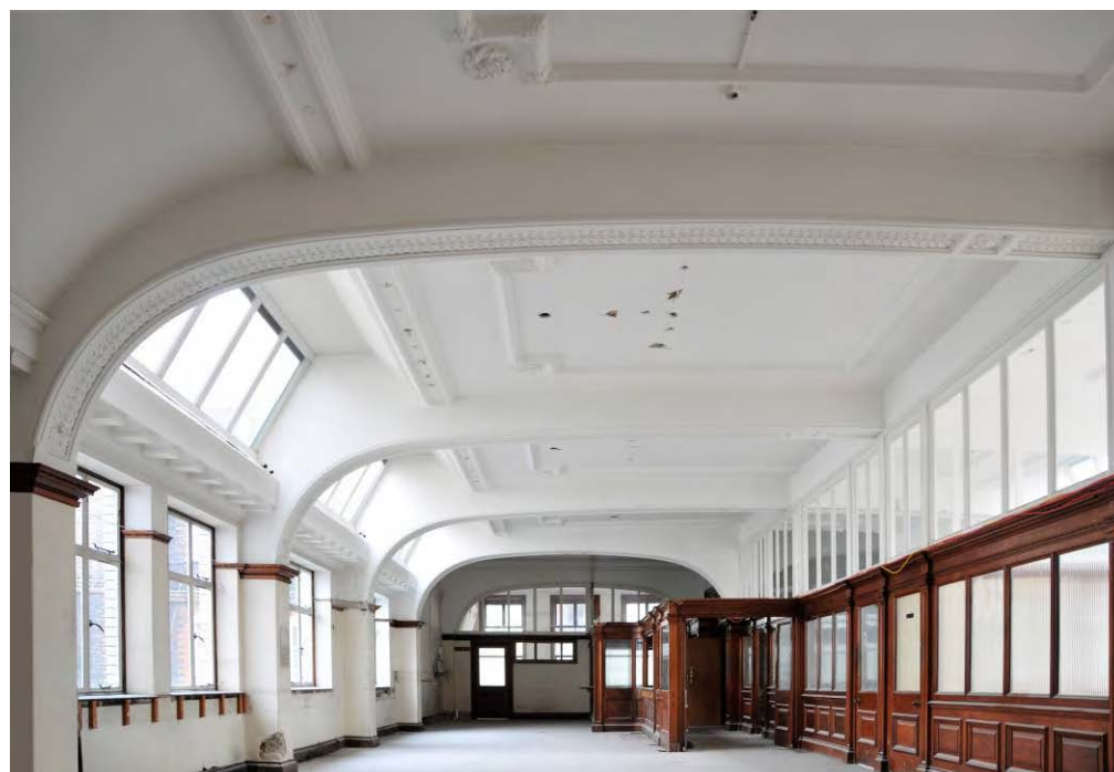
As existing perspective view of partitions from rear of main office space
