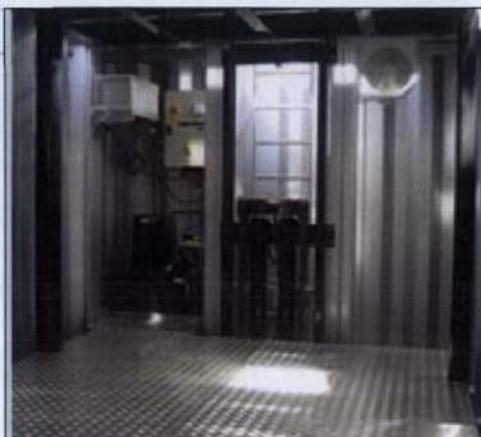
The power unit is situated in the service area.
