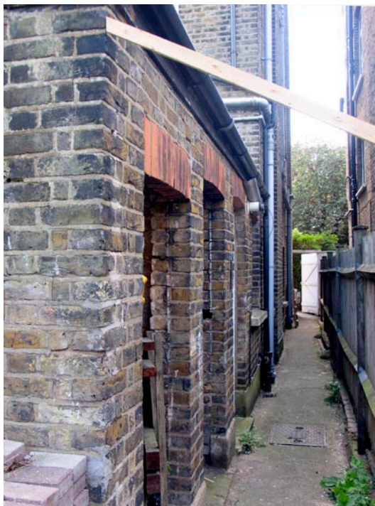
Left: Existing southwest elevation of rear annex Right: Existing northeast elevation of rear annex
