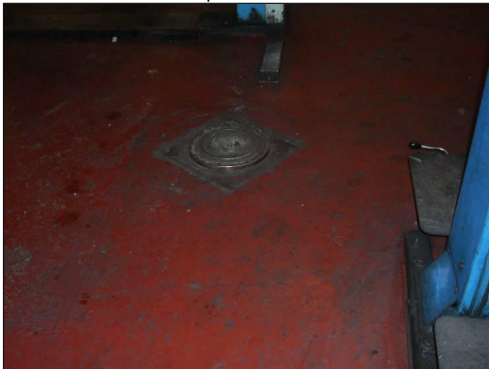
Photo 15. Evidence of potential UST
