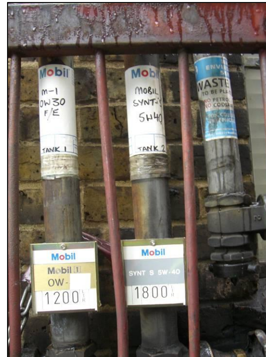
Photo 12. View of pipes used to fill AST tanks
