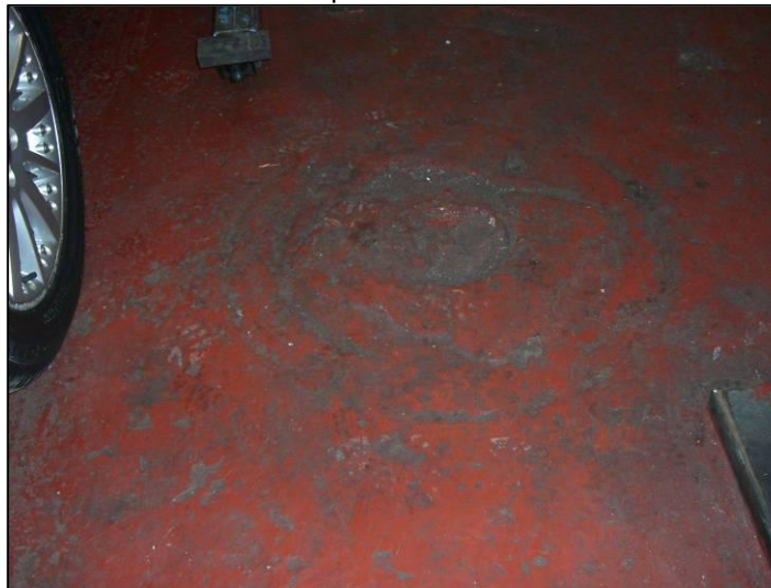
Photo 16. Evidence of potential UST
