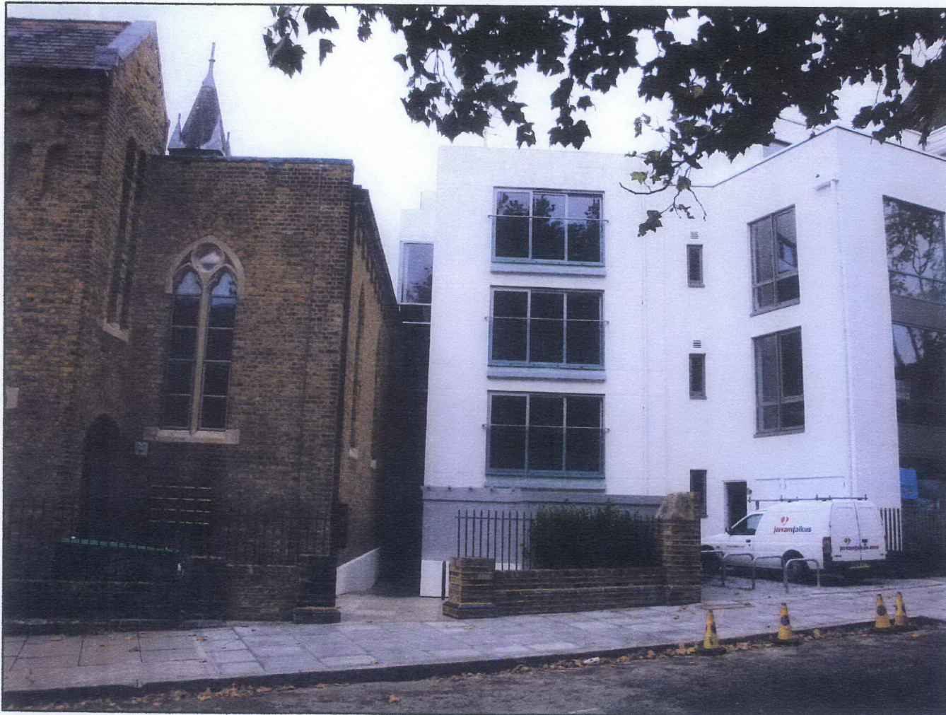
Front elevation view of window and curtain wall frame, render and downpipe
