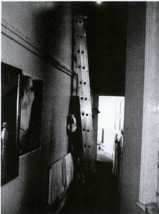
Photo #03 showing the proposed location of the new bedroom door in the area of the radiator and ladder.
