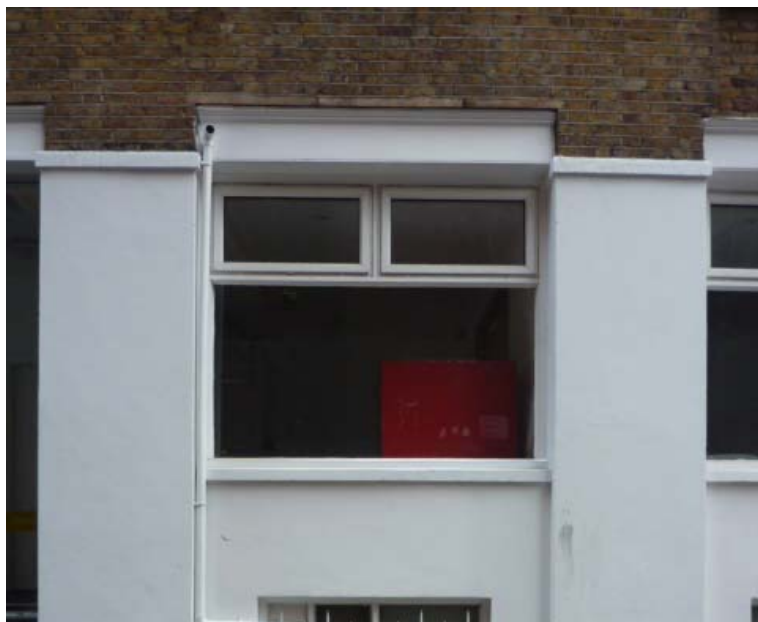
Image 7. The existing window arrangement is not original and not well executed.
