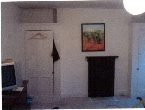
CUPBOARD AND PART OF SPINE WALL TO BE REMOVED TO ACCOMMODATE NEW BATHROOM
