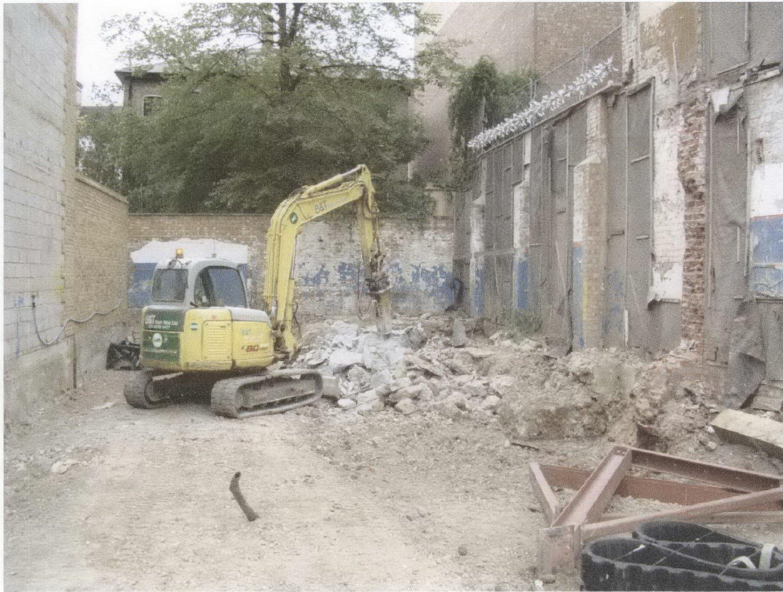
Approximately 500mm of made ground were removed and brought to a qualified disposal site.
