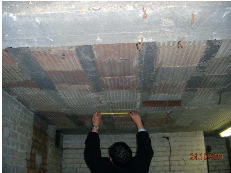
EXISTING ROOF SLAB CONSTRUCTED FROM REINFORCED CONCRETE BEAM RIBS SPACED APART BY HOLLOW CLAY POTS
