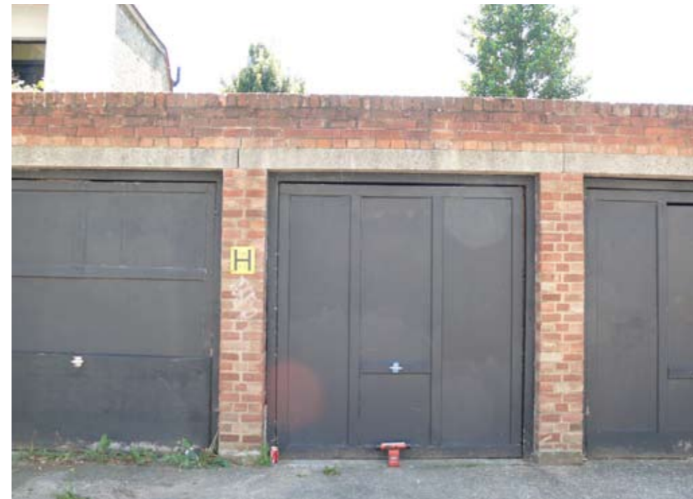
Low quality brick garages.
