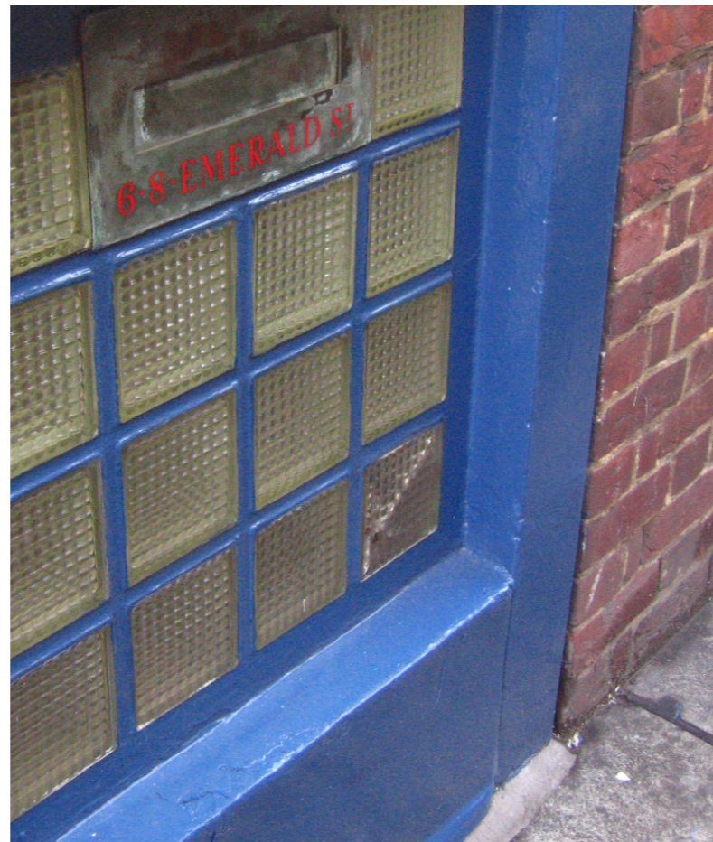
Existing glass blocks at low level are in poor state
