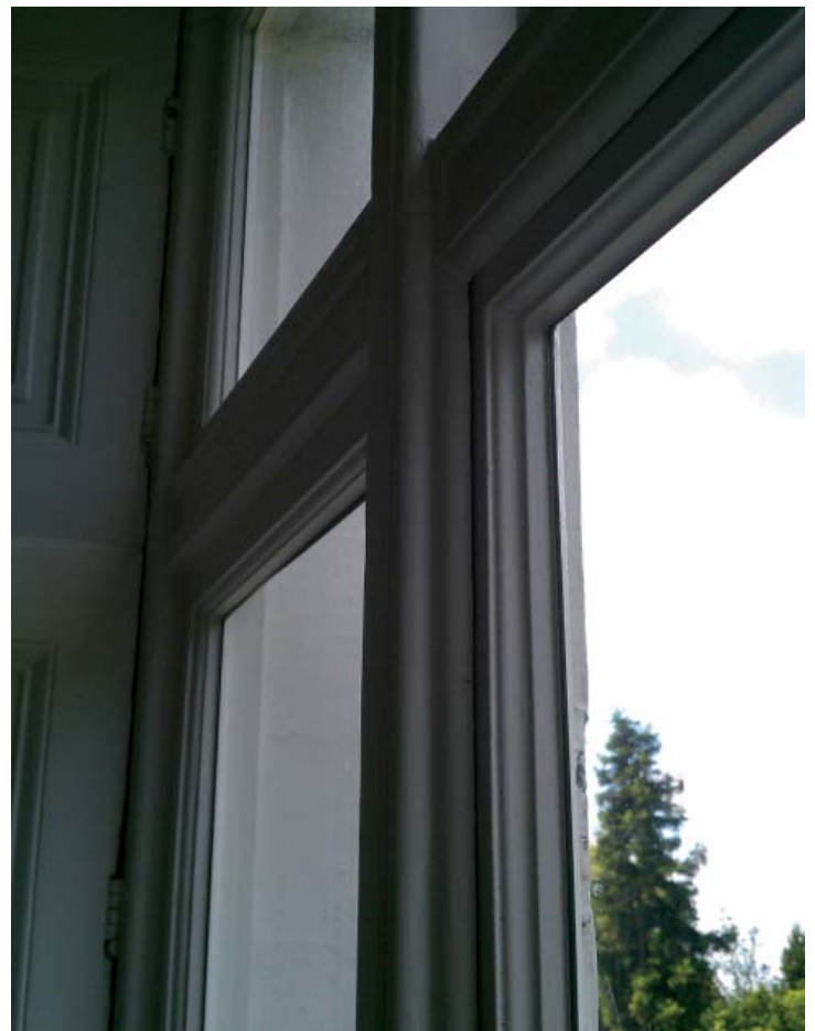
WINDOW W1.4- Rear single glazed. Original frame and original door door, modern flanking fixed panels
