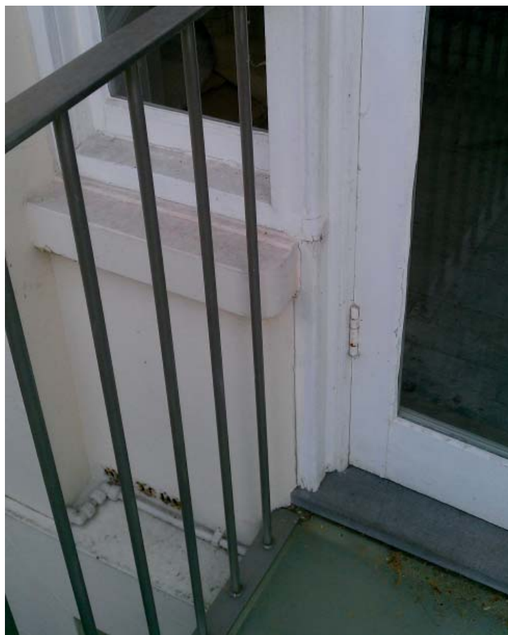
WINDOW WG.4- Frame cut when door was installed
