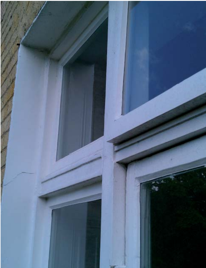
WINDOW W1.4- Rear single glazed. Original frame and original door door, modern flanking fixed panels
