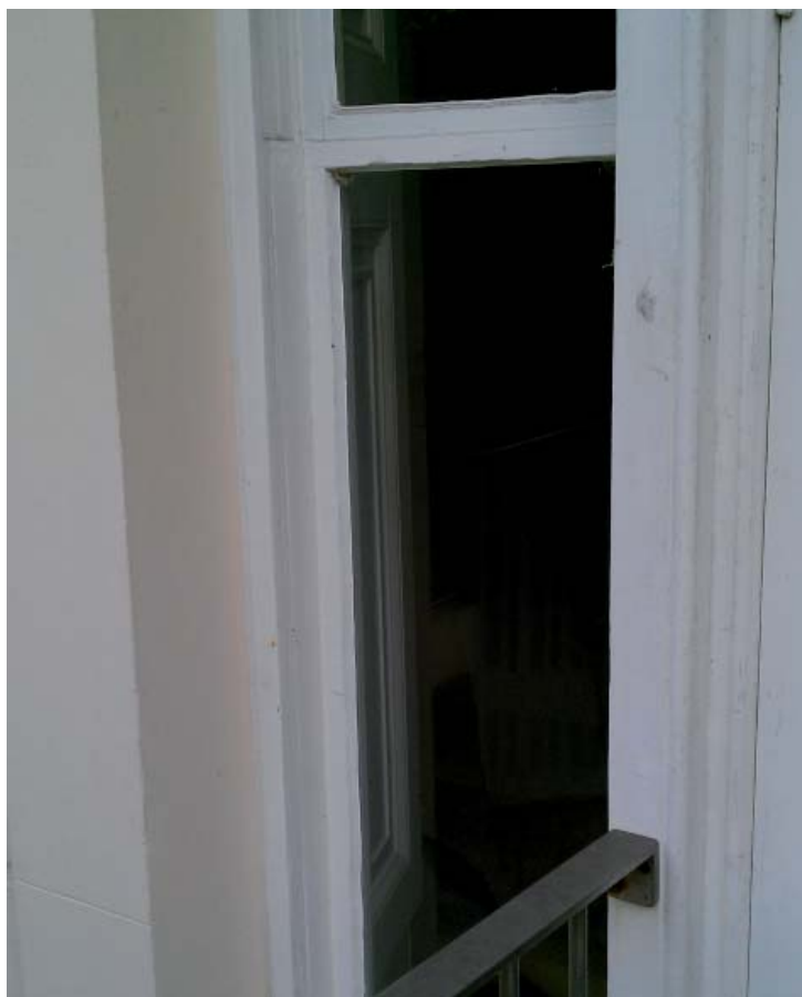
WINDOW WG.4- Rear single glazed Blocked sashes
