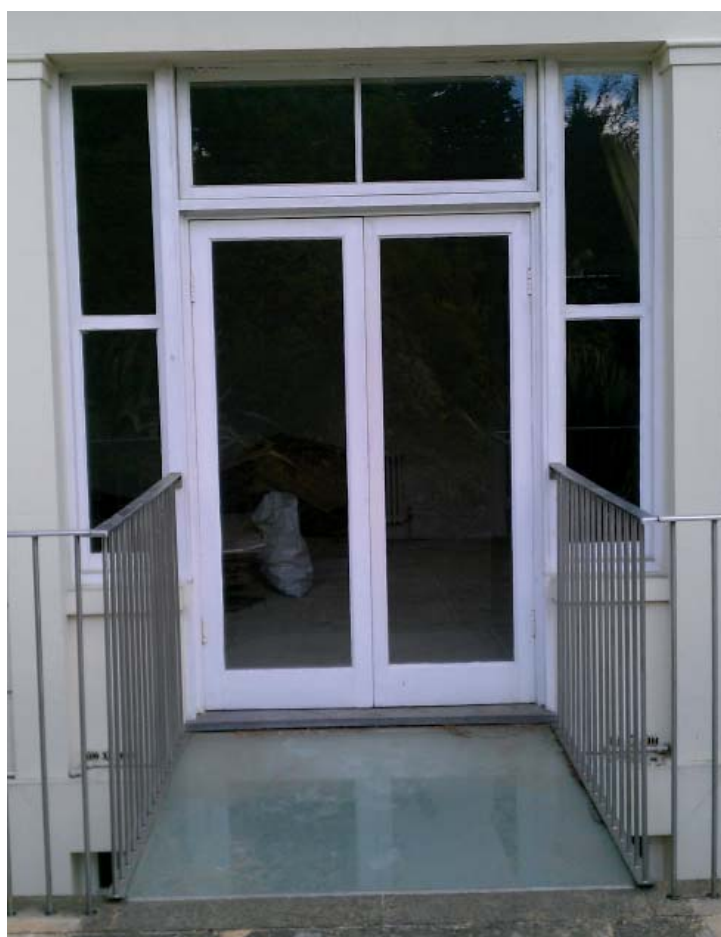
WINDOW WG.4- Rear single glazed. Original frame and Modern door, modern blocked sashes
