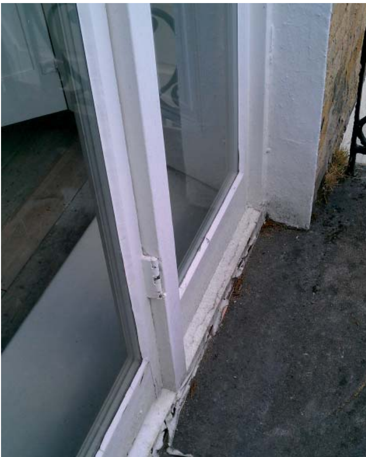
WINDOW WG.4- Rear single glazed. Original frame and original door door, modern flanking fixed panels
