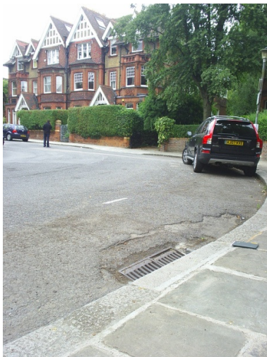
Figure 1 Lowest Point in Road looking looking towards 16a Driveway
