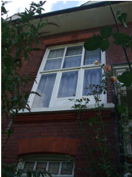
Existing window to be replaced with new Window matching the original (no 18).
