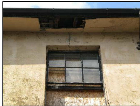
Failure of the original lath & plaster at eaves level
