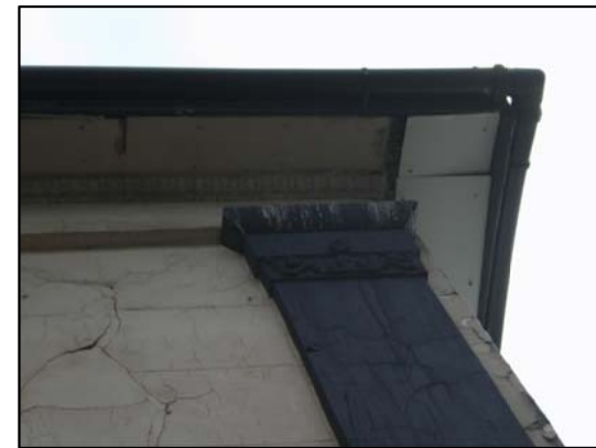
Failure of the original lath and plaster lead to the use of plywood boards to cover the exposed roof structure
