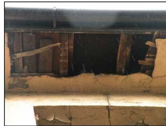
Close-up of the failed lath & plaster showing exposed rafters
