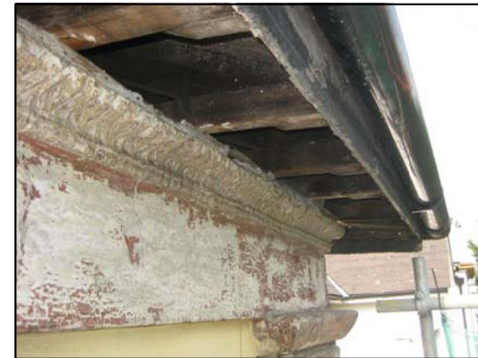
Failure of the lath & plaster eaves resulted in some water ingress that lead to some minor damage to the roof structure
