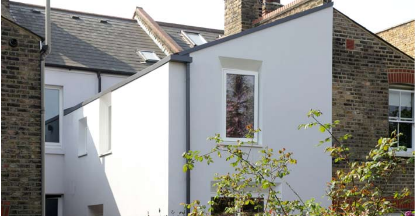
An example of a rendered external wall insulation installation. The gutter and verge have been extended to protect the insulation and provide a simple neat interface between the wall and roof.
