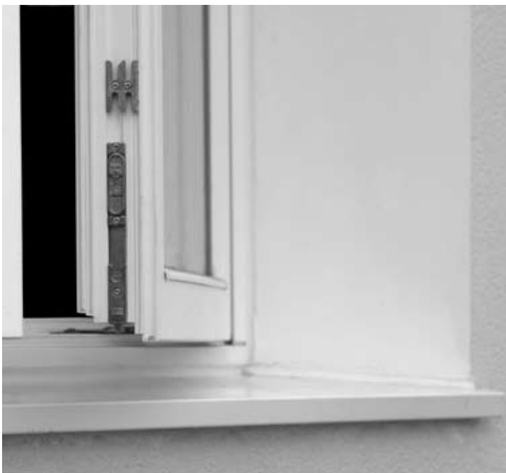
An example of a high quality triple glazed window fitted within a wall insulated externally with rendered insulation.
