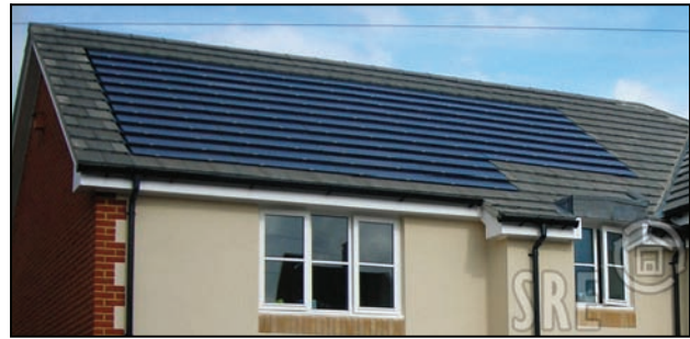
Building Integrated PV Array (Tile)
