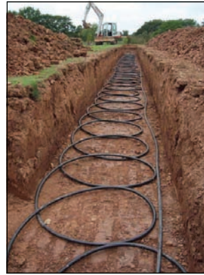
External Collection Trench
