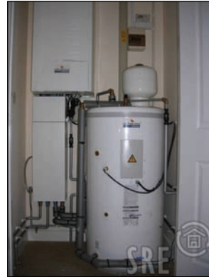
Internal Control Unit and Thermal Store
