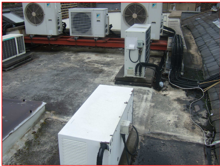
EXISTING CONDENSER MOUNTED ON EXISTING CONCRETE PLATFORM
