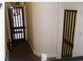
Inappropriate door to G2 to be replaced by new Type 'A' internal door and existing screen between inner/outer hallways to be removed
