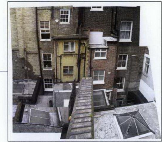
All unsympathetic later ground level additions to be removed to return properties and plan forms to their historic character, layout and use. Unsightly modern red brick / render turret to be removed
