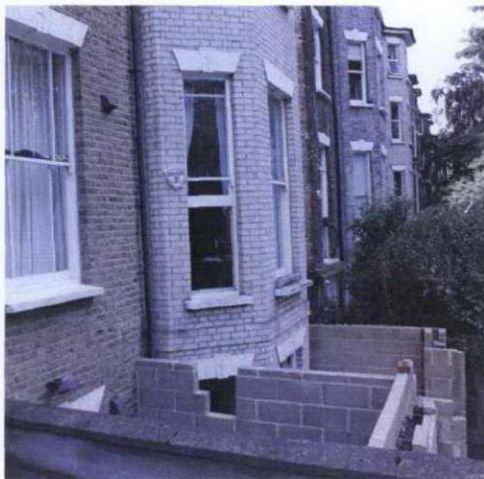
Rear elevation showing existing windows and the new lower ground floor extension.
