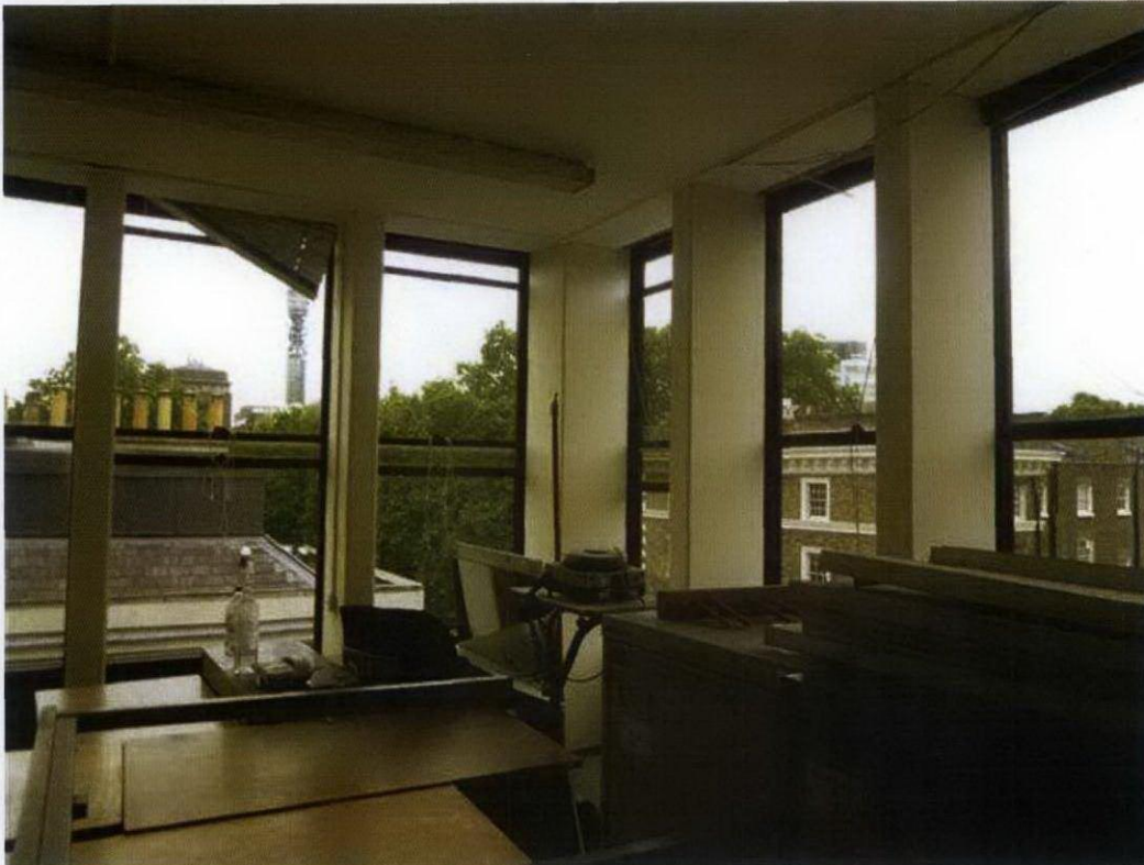
3: Corner office showing existing decorated exposed mullions & exposed soffit (to be retained)
