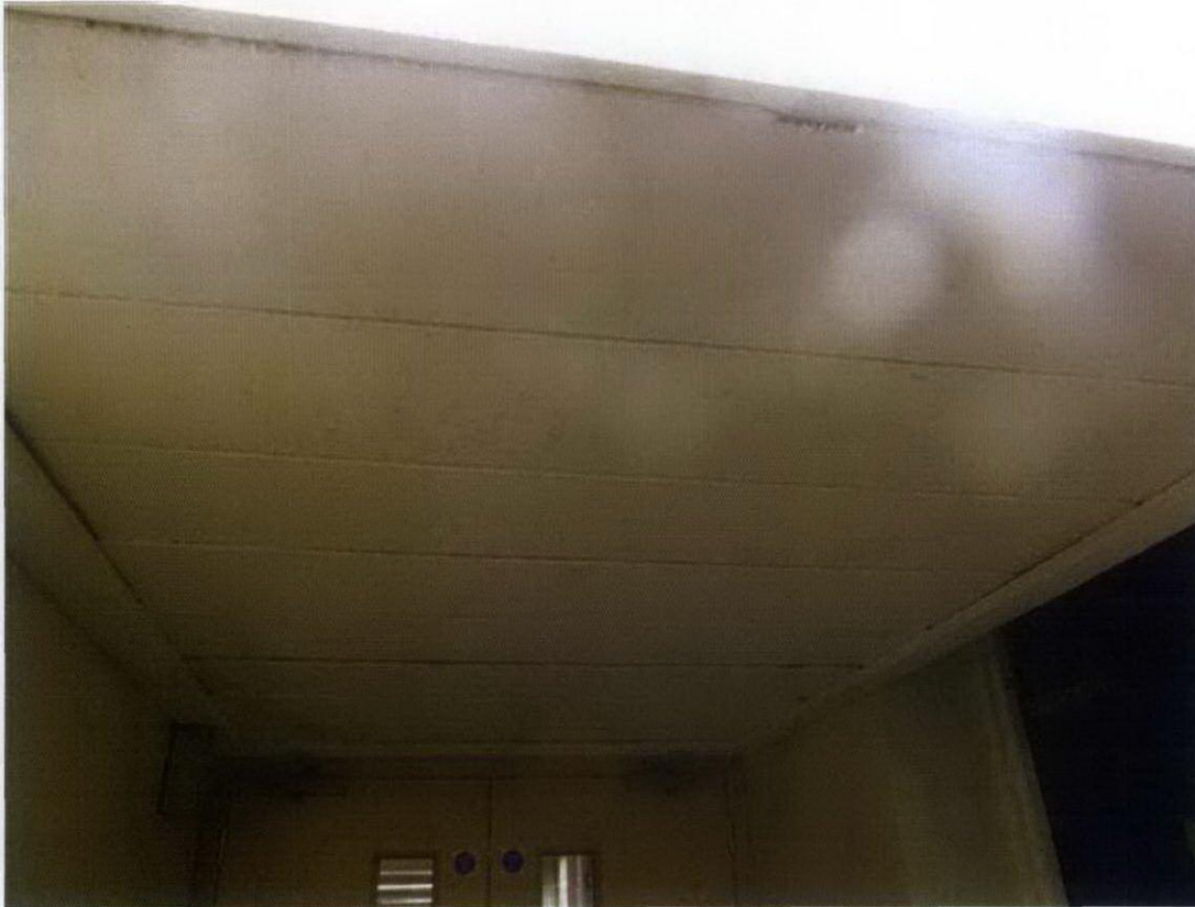
5: Existing plank ceiling to be removed within works areas. To be removed & reinstated within lift lobby area.
