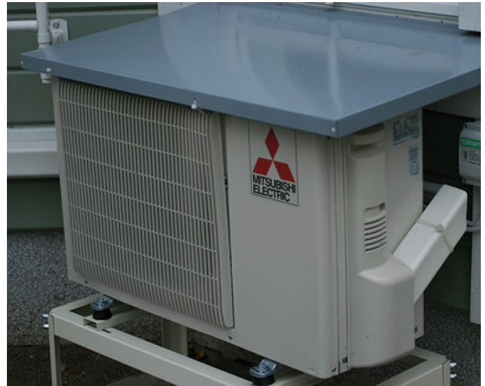
ASHP external unit
